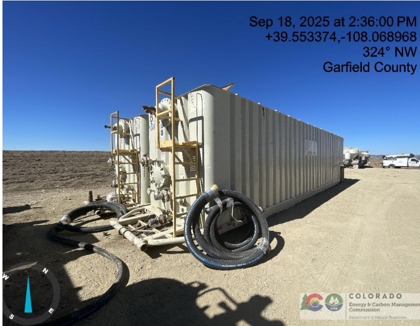
Photo # 1156 Frac tanks lack required labeling
