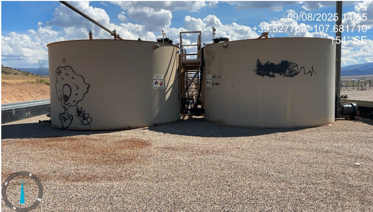
Photo 6: Graffiti appears to be present on tanks at the location.
