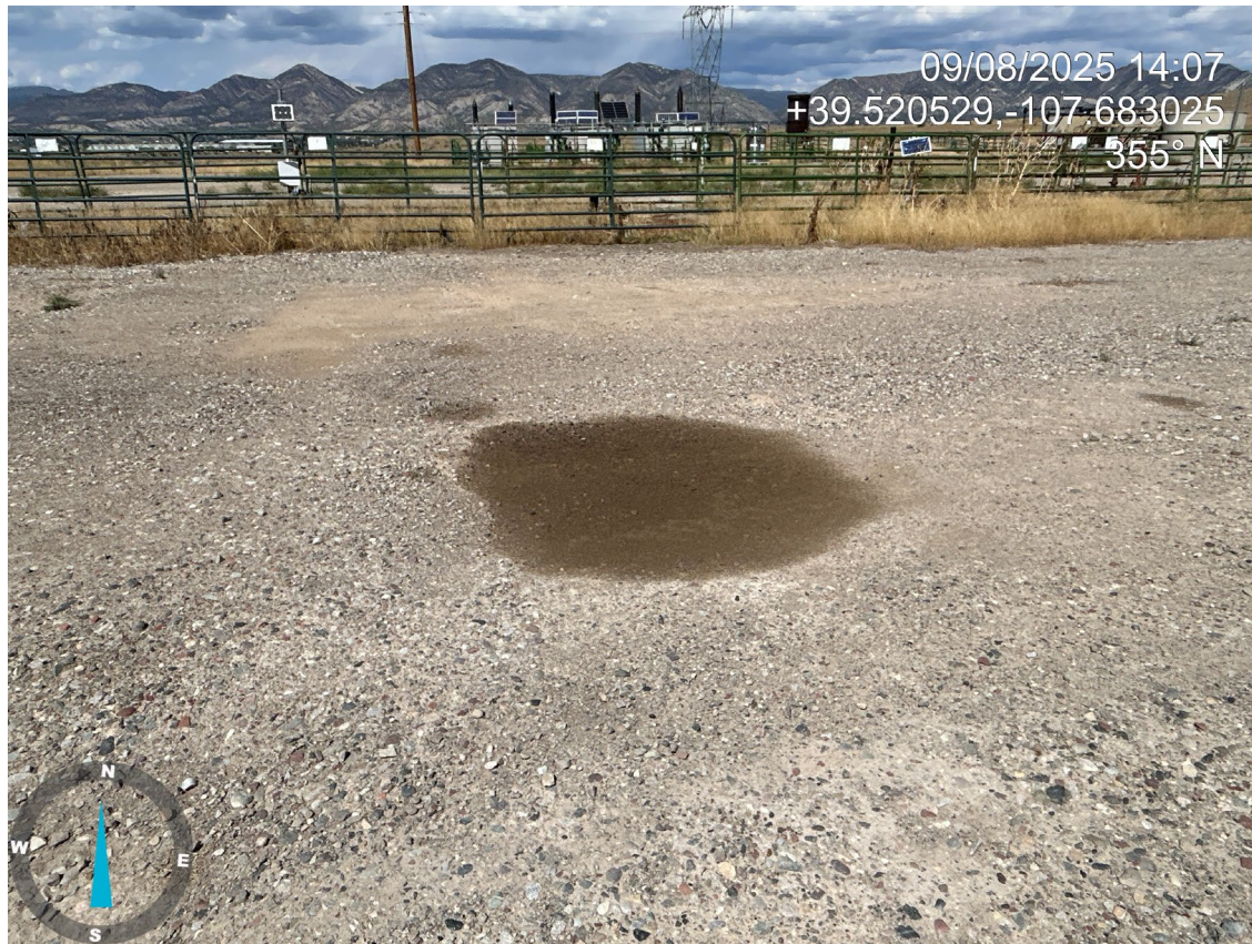
Photo 4: Staining is present on the working pad surface near the wellheads. Comply with Rule 912.a.
