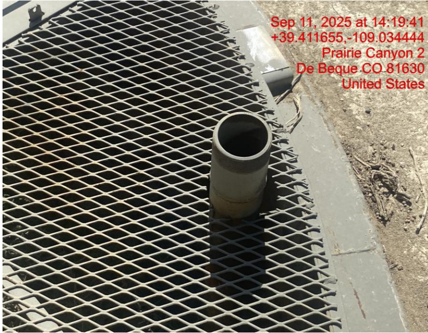
Open-Ended Line/Wildlife Entry Hazard on Tank Screen – Photo #00713
