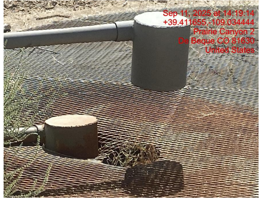
Wildlife Entry Hazard on Tank Screen – Photo #00712
