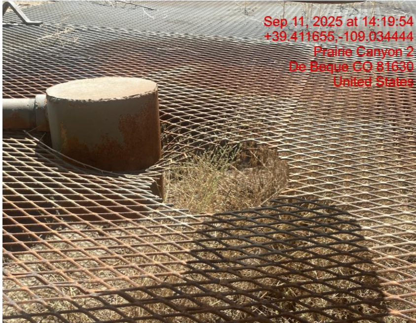
Wildlife Entry Hazard on Tank Screen – Photo #00714
