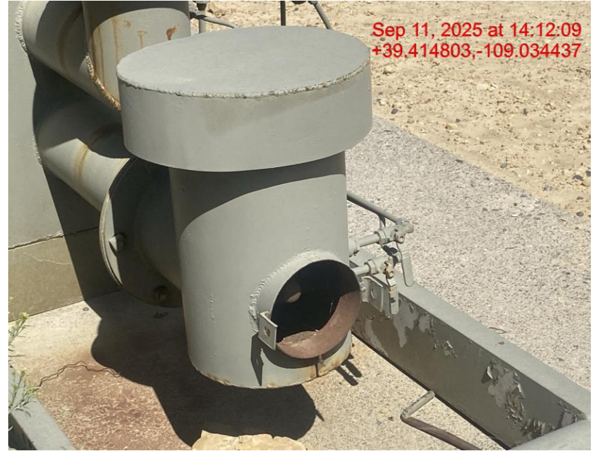
Wildlife Entry Hazard – Photo #00702
