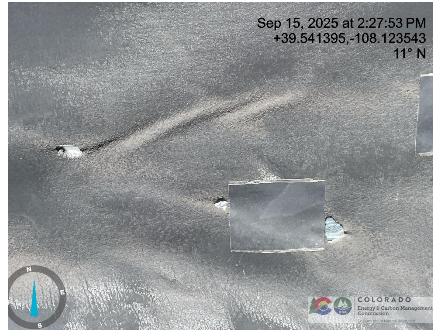
Photo # 9378 Holes in secondary containment liner/liner needs maintenance
