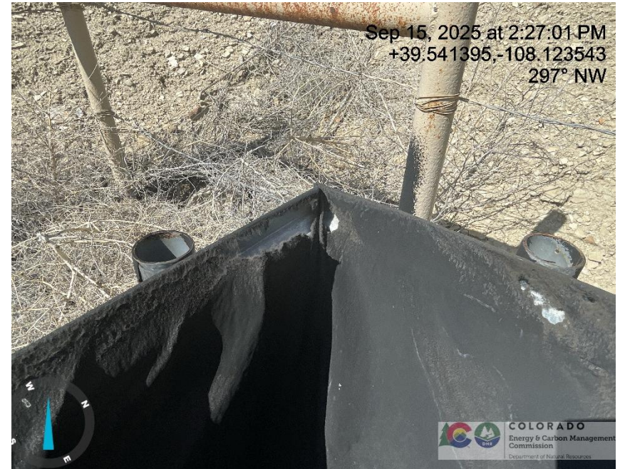
Photo # 9380 Holes in secondary containment liner/liner needs maintenance
