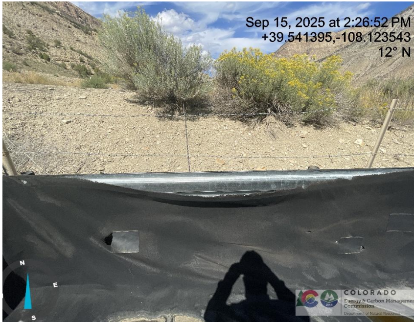
Photo # 9381 Secondary containment liner damaged/liner needs maintenance
