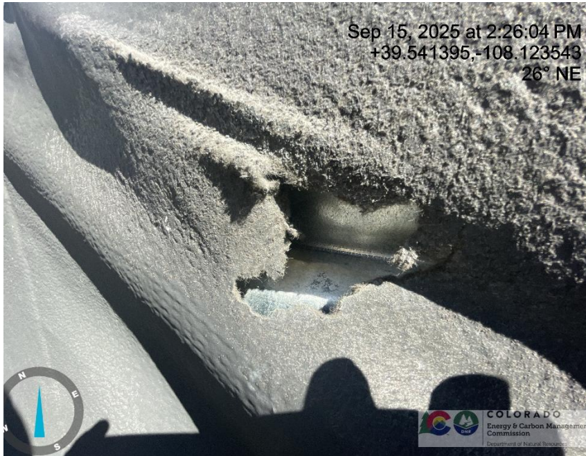
Photo # 9383 Hole in secondary containment liner/liner needs maintenance
