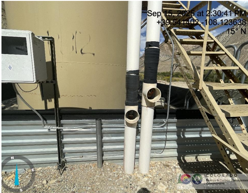
Photo # 9375 Flowline heating insulation open ended /wildlife hazard/available for entry by wildlife
