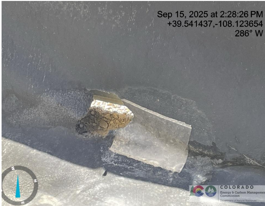
Photo # 9377 Hole in secondary containment liner/liner needs maintenance
