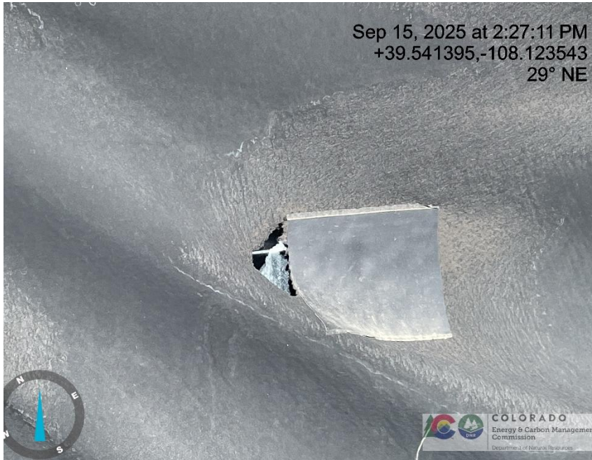
Photo # 9379 Hole in secondary containment liner/liner needs maintenance
