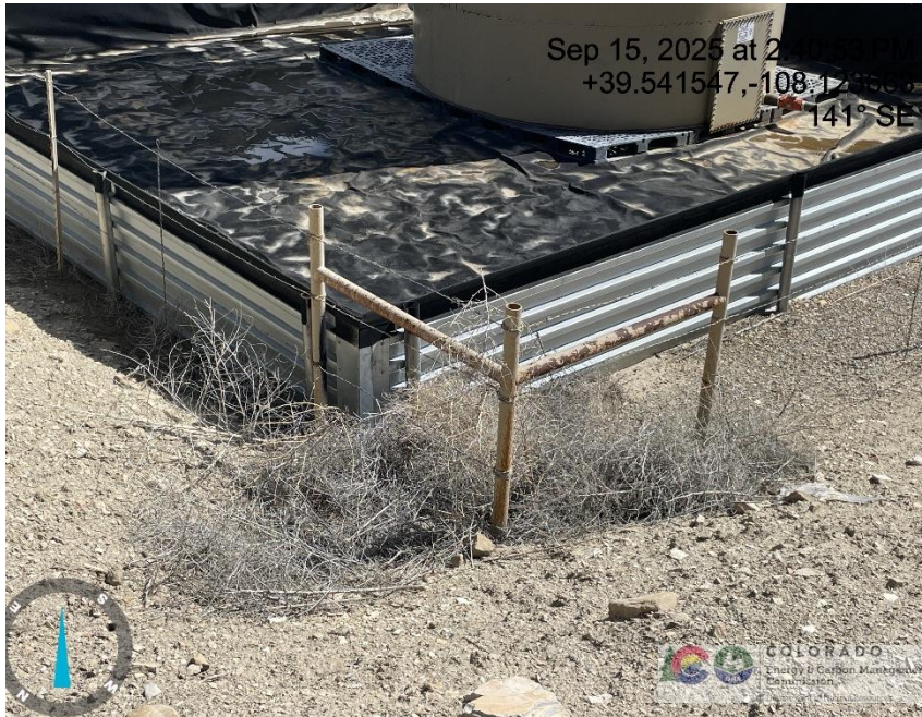
Photo # 9385 Dead weeds/debris
