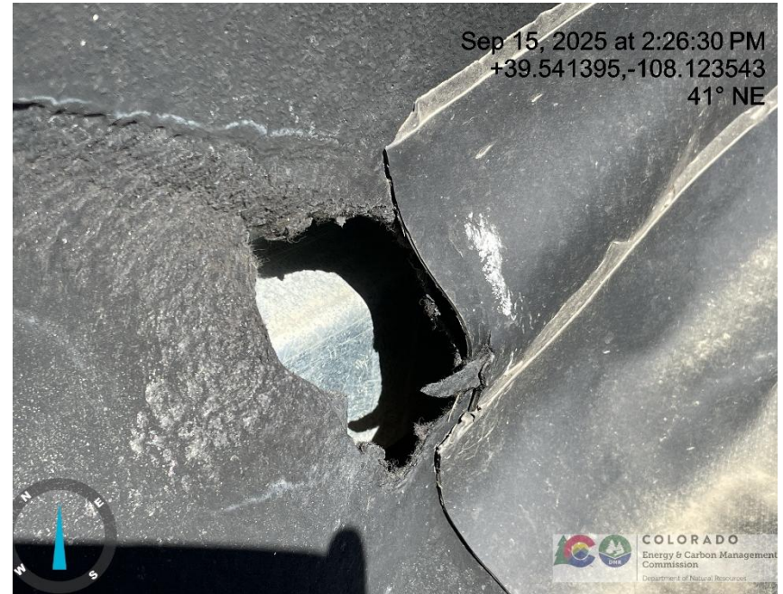
Photo # 9382 Hole in secondary containment liner/liner needs maintenance
