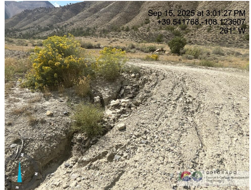
Photo # 9405 Erosion & transport of sediment on lease road /insufficient BMP's
