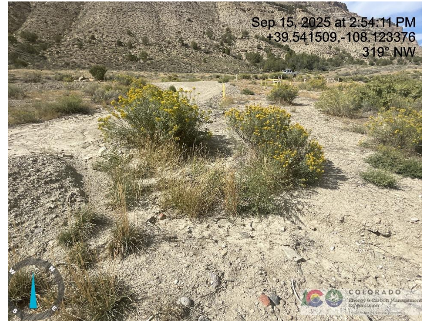
Photo # 9397 Erosion & transport of sediment on lease road & going off lease road into a vegetated area/insufficient BMP's
