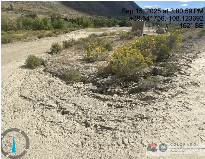
Photo # 9404 Erosion & transport of sediment on lease road /insufficient BMP's
