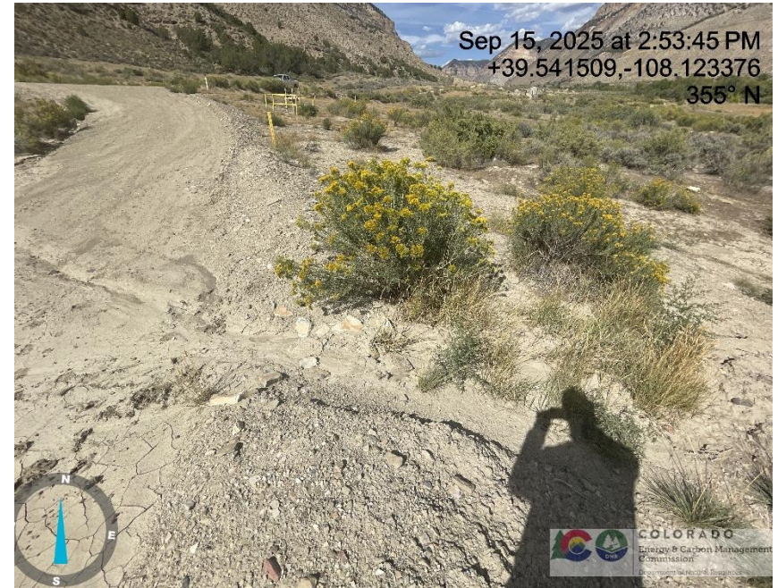
Photo # 9393 Erosion & transport of sediment on lease road & going off lease road into a vegetated area/insufficient BMP's
