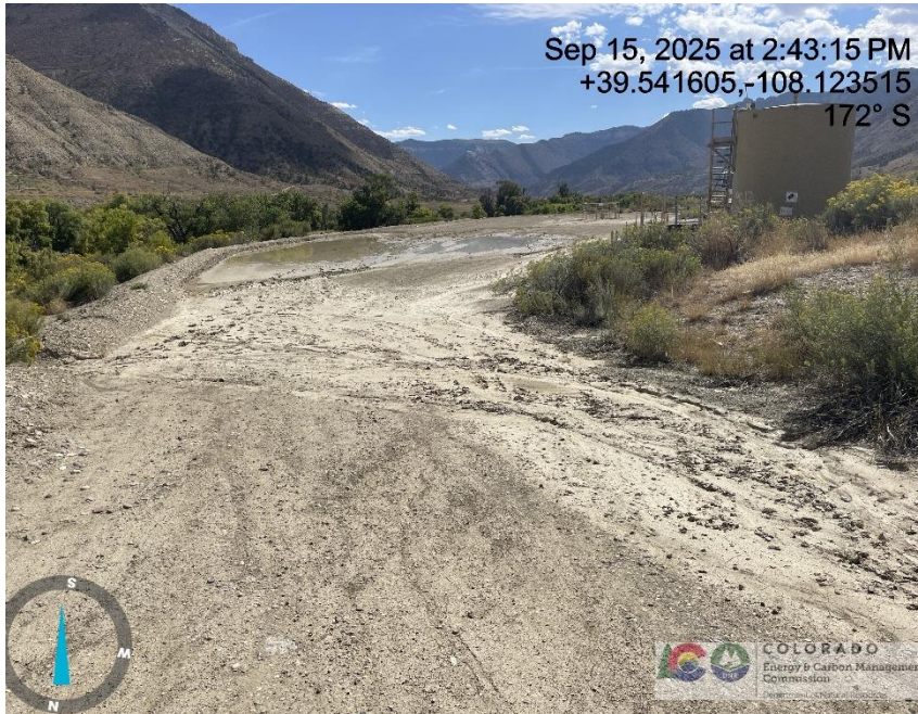
Photo # 9390 Erosion & transport of sediment on lease road & onto location/insufficient BMP's
