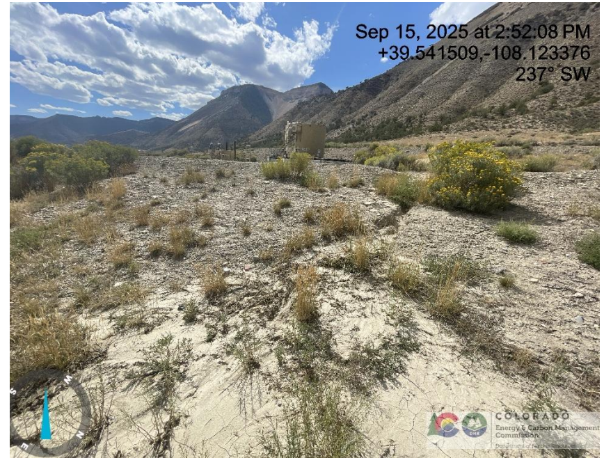
Photo # 9401 Erosion & transport of sediment off lease road & into a vegetated area/insufficient BMP's
