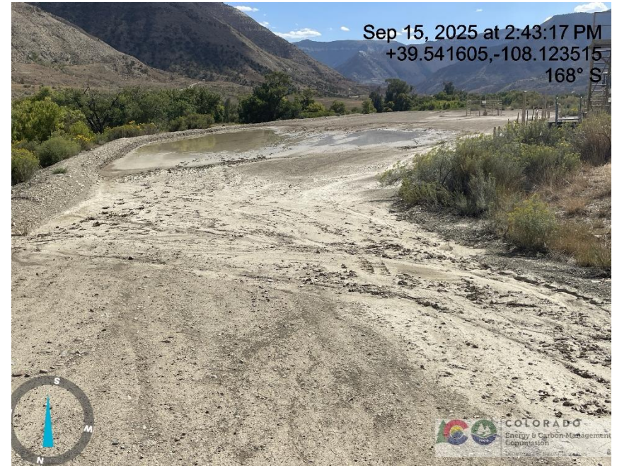
Photo # 9391 Erosion & transport of sediment on lease road & onto location/insufficient BMP's
