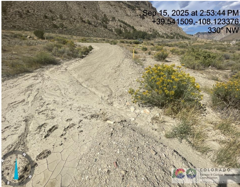
Photo # 9392 Erosion & transport of sediment on lease road & going off lease road into a vegetated area/insufficient BMP's
