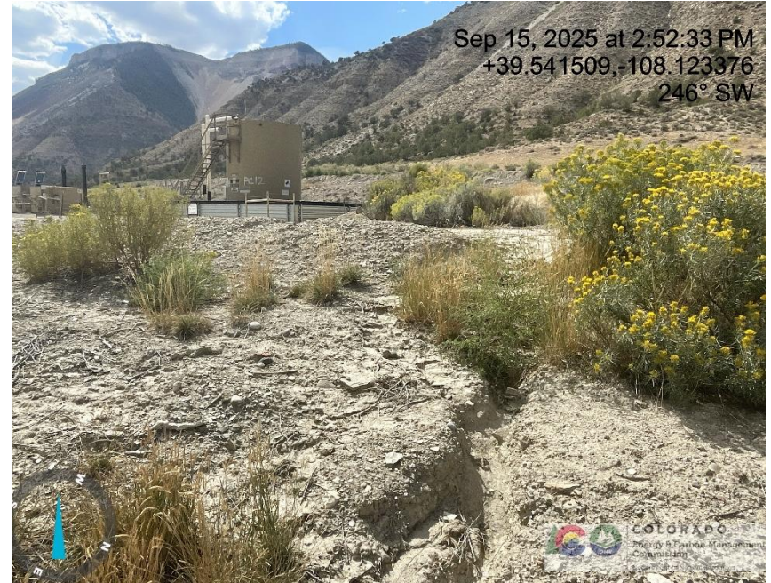
Photo # 9399 Erosion & transport of sediment off lease road & into a vegetated area/insufficient BMP's
