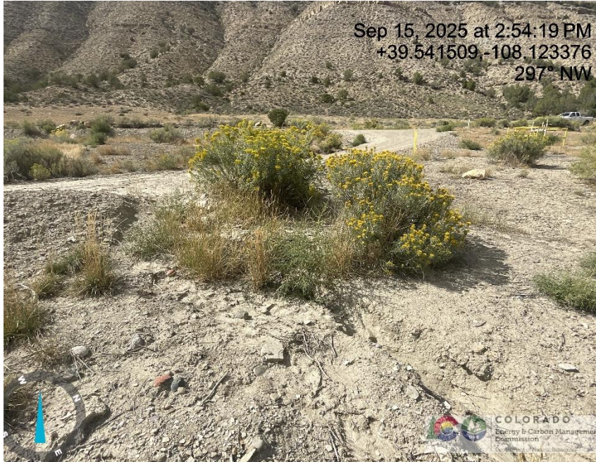
Photo # 9398 Erosion & transport of sediment off lease road & into a vegetated area/insufficient BMP's
