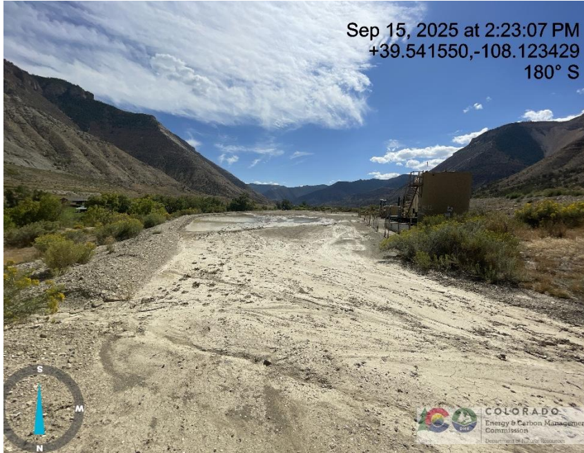
Photo # 9386 Erosion & transport of sediment on lease road & onto location/insufficient BMP's
