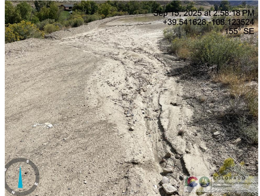
Photo # 9387 Erosion & transport of sediment on lease road & onto location/insufficient BMP's
