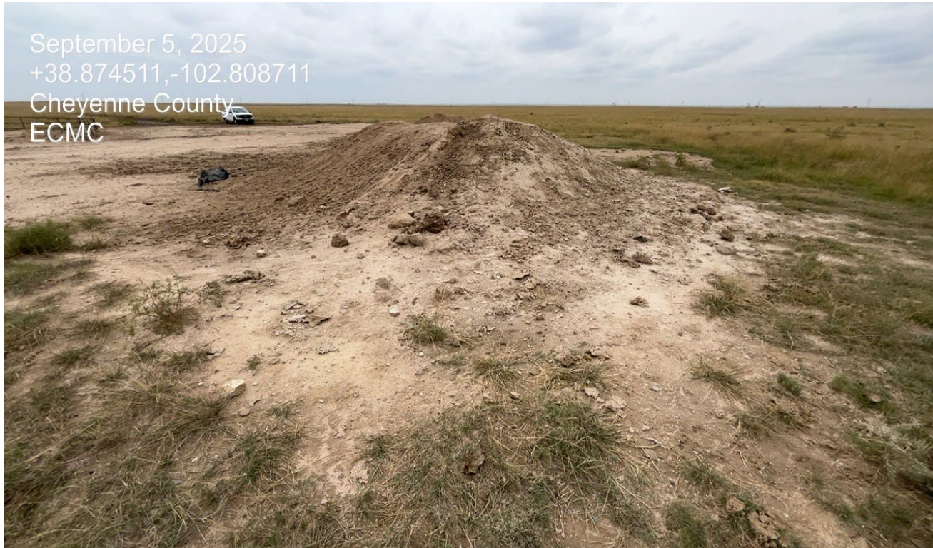
Photo 6 . Facing northeast. The excavated impacted material was placed on a piece of plastic with no containment and some of the material has fallen outside of the liner. The plastic was also torn and compromised.
