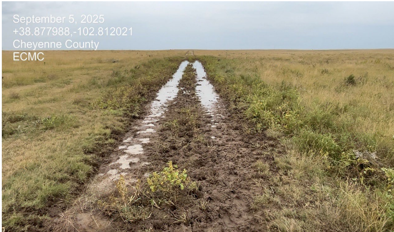
Photo 1. Facing southeast toward the access road. The access road is impassible due to stormwater accumulating along the road. Since the well has been PA'd the road will need to be decompacted, regraded, and reclaimed.
