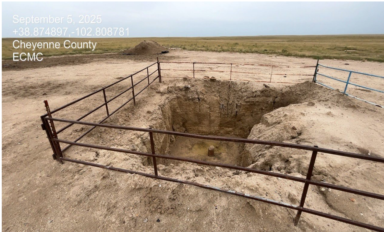
Photo 3. Facing toward the cut/capped wellhead. Contaminated material has been excavated from the wellhead and placed at the southeast side of the location.
