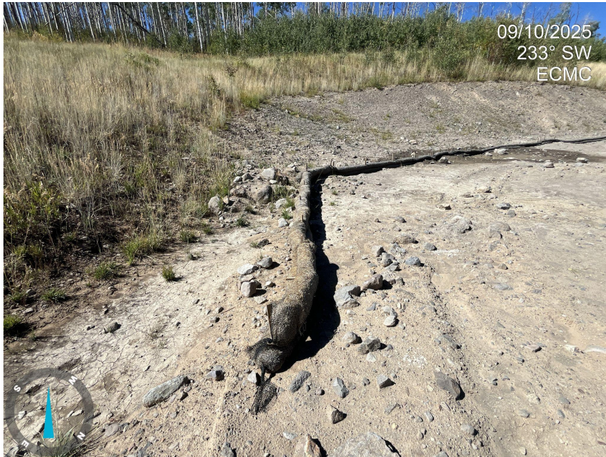
Photo 1. Photos 1-5 taken at the southeastern portion of the Location, near the cut slope where the cuttings waste was stored. Photos illustrate that stormwater BMPs are no longer functioning per good engineering practices. Stormwater has commingled with cuttings material and has moved onto the pad.
