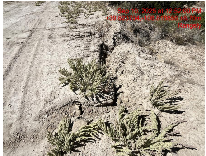
Photo # 3126 Failure to minimize erosion & transport of sediment off location/insufficient BMP's
