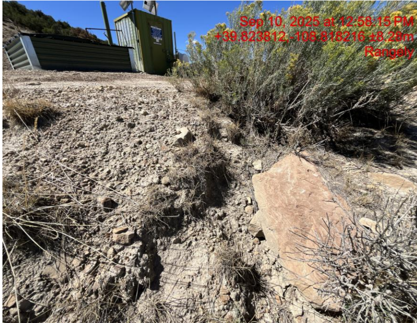
Photo # 3132 Failure to minimize erosion & transport of sediment off location/insufficient BMP's
