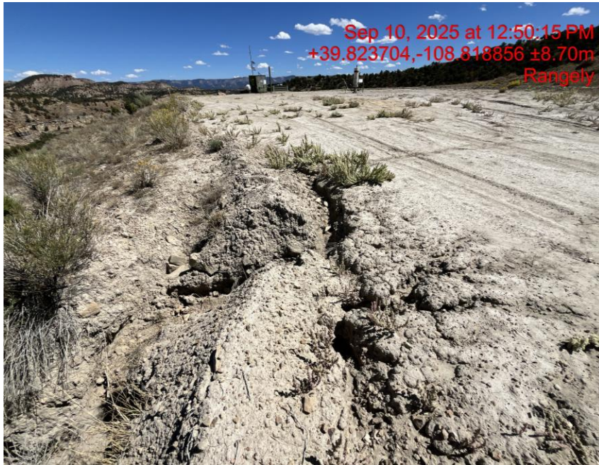
Photo # 3124 Failure to minimize erosion & transport of sediment off location/insufficient BMP's
