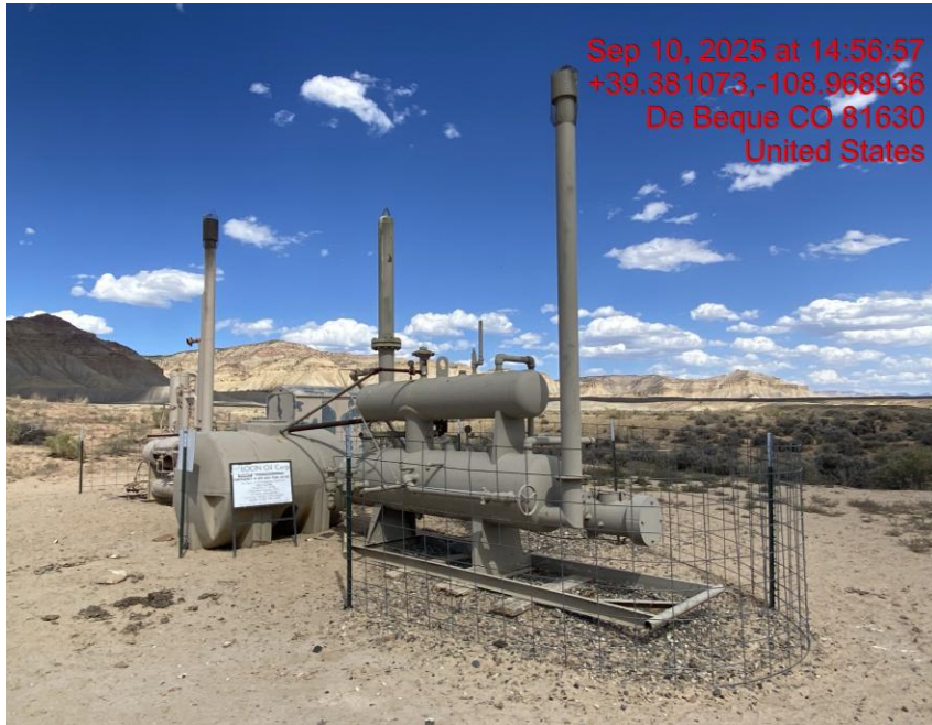
Location/No Secondary Containment for Chemical Tank – Photo #00687
