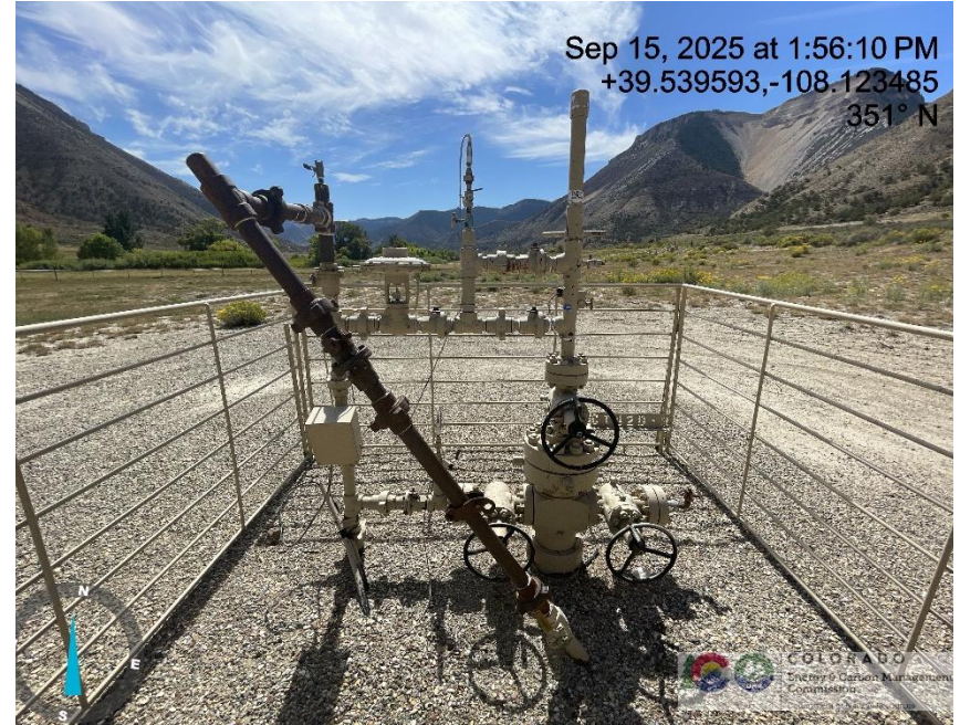
Photo # 9232 Bradenhead line tied into flowline/no FORM 4 SUNDRY
