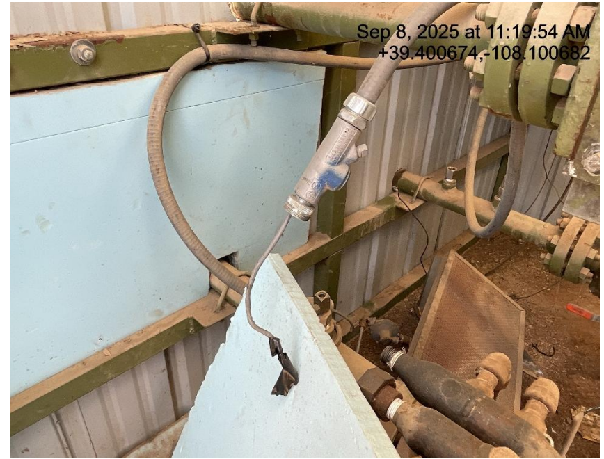
Photo # 6378 Wiring for gas meter disconnected/meter not in use
