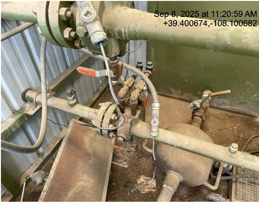
Photo # 6377 Wiring for gas meters disconnected/meters not in use
