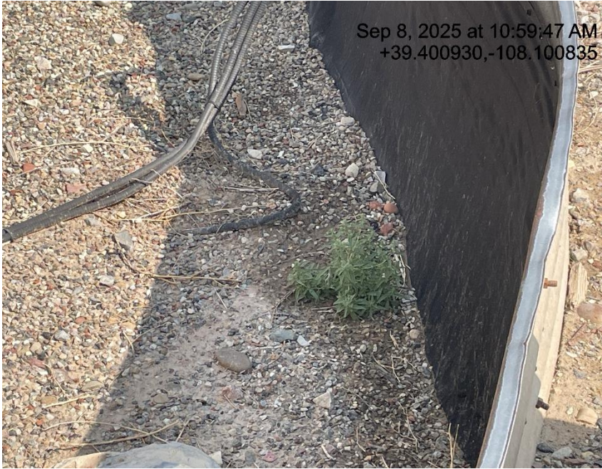
Photo # 6379 Weeds in secondary containment
