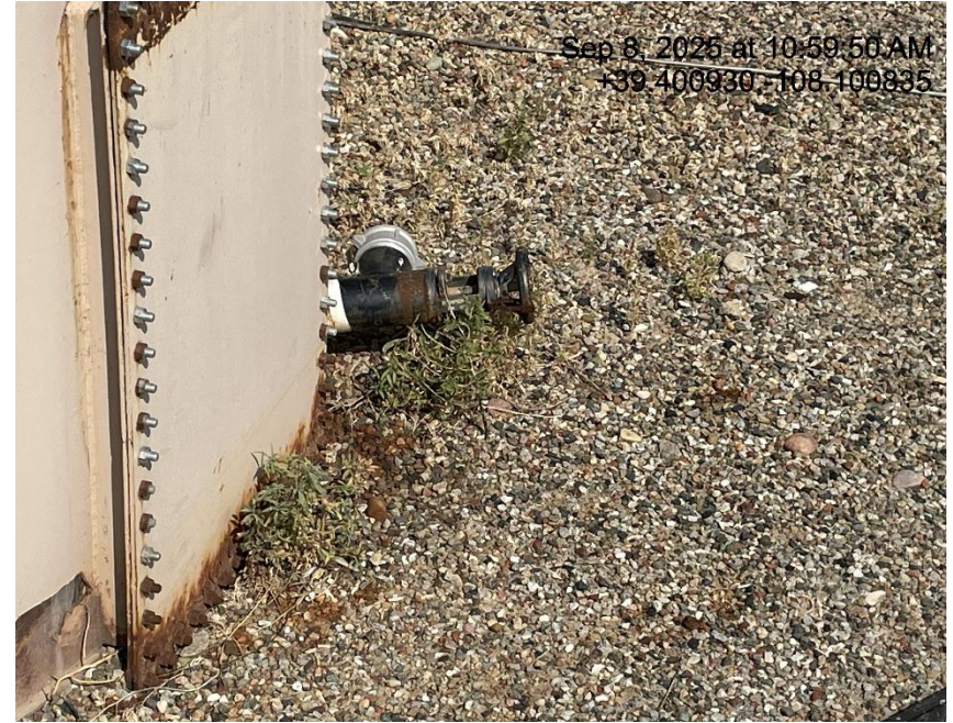
Photo # 6380 Weeds in secondary containment
