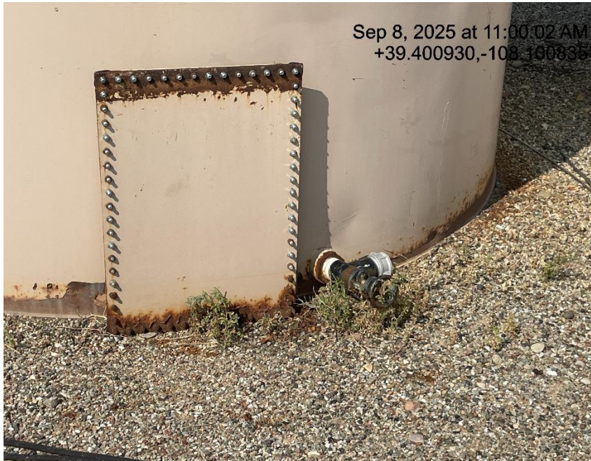
Photo # 6381 Weeds in secondary containment
