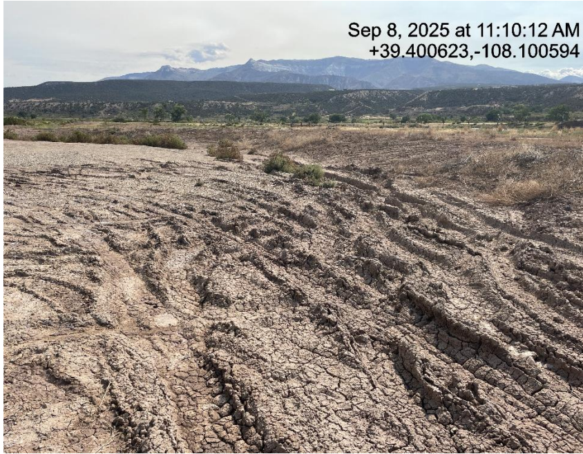
Photo # 6384 Lack of stabilization/compaction on location
