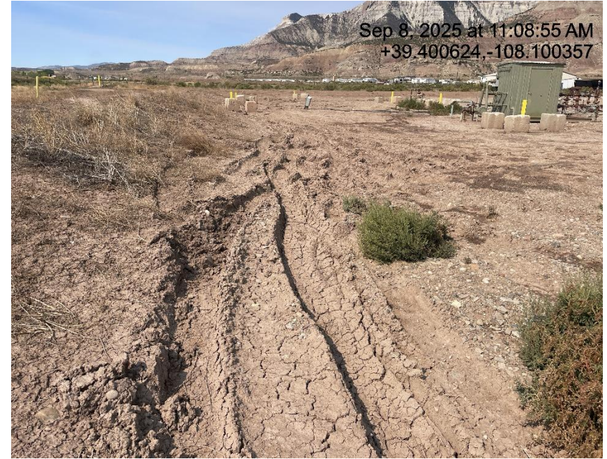
Photo # 6385 Lack of stabilization/compaction on location
