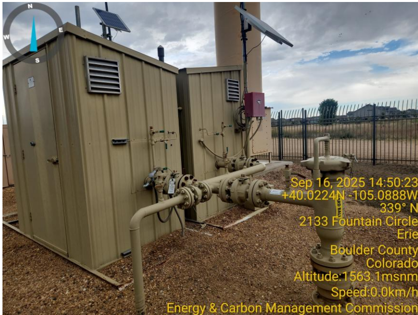
Photo 7 Gas Meter Run x 2.
