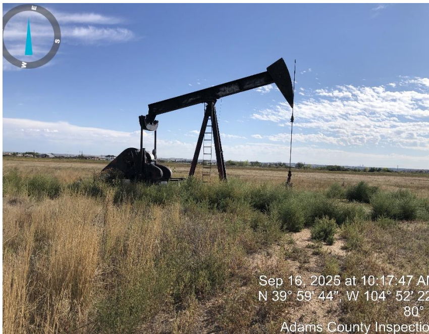
Photo#1 Pumpjack/Weeds around pumpjack have not been addressed from Document#717000452
