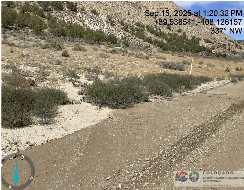
Photo # 8543 Erosion & transport of sediment onto lease road/insufficient BMP's (approximately 3/10th of a mile from entrance to location)
