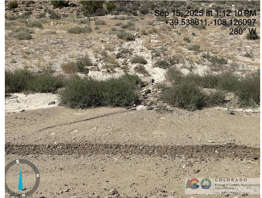
Photo # 8534 Erosion & transport of sediment onto lease road/insufficient BMP's (approximately 3/10th of a mile from entrance to location)
