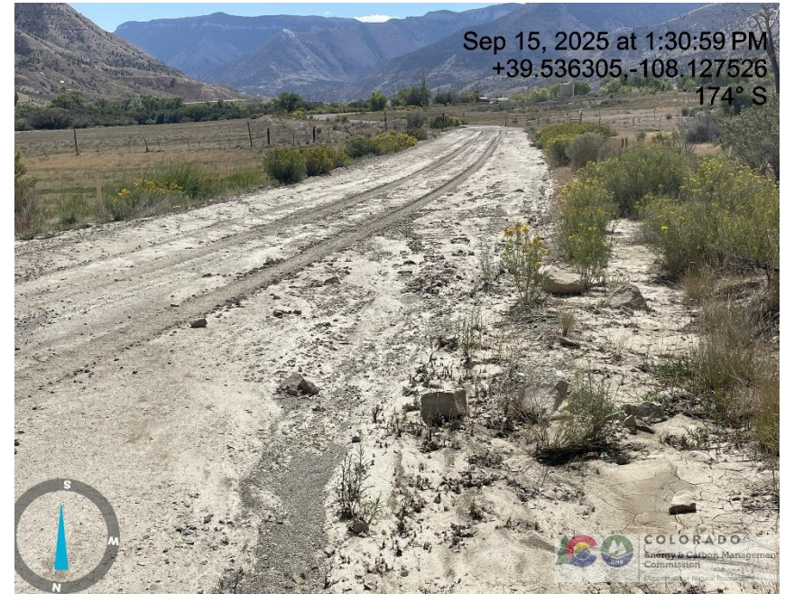
Photo # 8564 Erosion & transport of sediment onto lease road/insufficient BMP's (approximately 6/10th of a mile from entrance to location)
