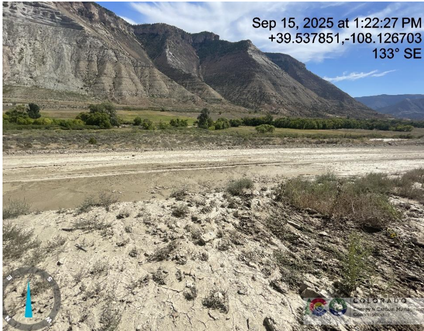
Photo # 8549 Erosion & transport of sediment onto lease road/insufficient BMP's (approximately 4/10th of a mile from entrance to location)
