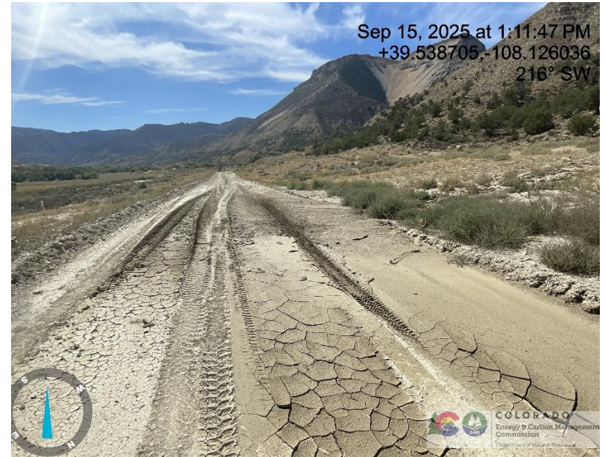
Photo # 8530 Erosion & transport of sediment onto lease road/insufficient BMP's (approximately 3/10th of a mile from entrance to location)
