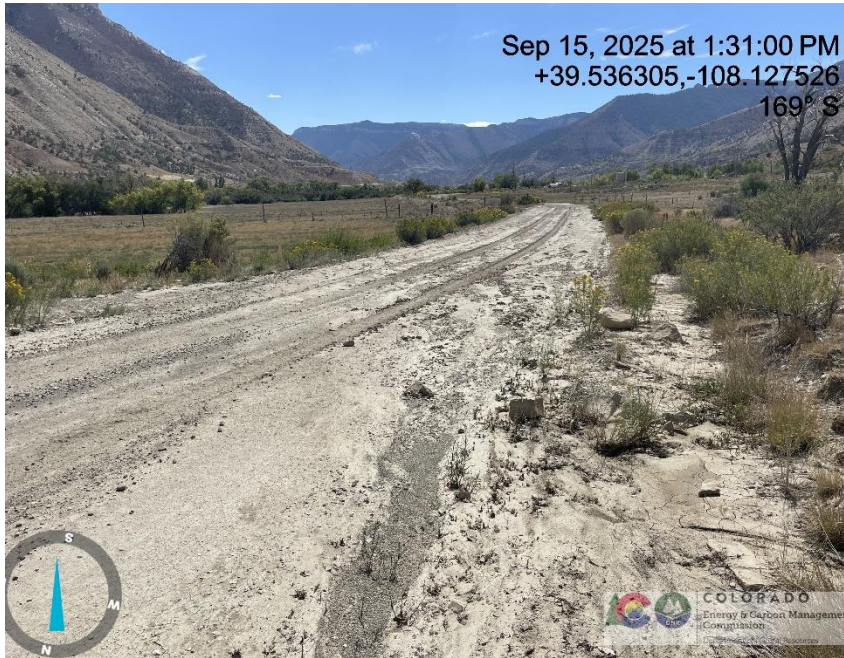
Photo # 8563 Erosion & transport of sediment onto lease road/insufficient BMP's (approximately 6/10th of a mile from entrance to location)
