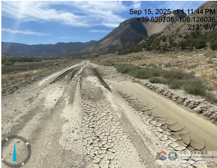
Photo # 8529 Erosion & transport of sediment onto lease road/insufficient BMP's (approximately 3/10th of a mile from entrance to location)
