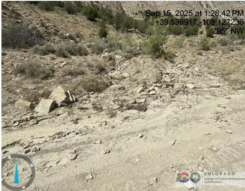
Photo # 8561 Erosion & transport of sediment onto lease road/insufficient BMP's (approximately 5/10th of a mile from entrance to location)
