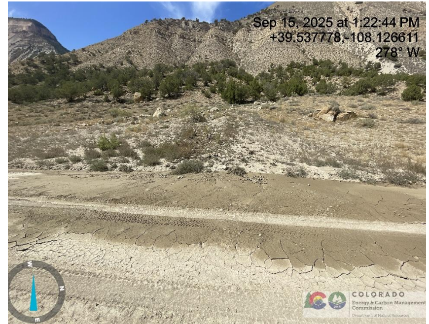
Photo # 8550 Erosion & transport of sediment onto lease road/insufficient BMP's (approximately 4/10th of a mile from entrance to location)
