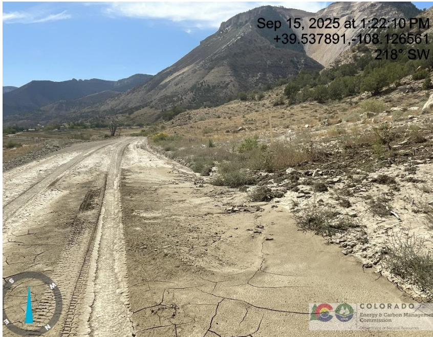
Photo # 8547 Erosion & transport of sediment onto lease road/insufficient BMP's (approximately 4/10th of a mile from entrance to location)
