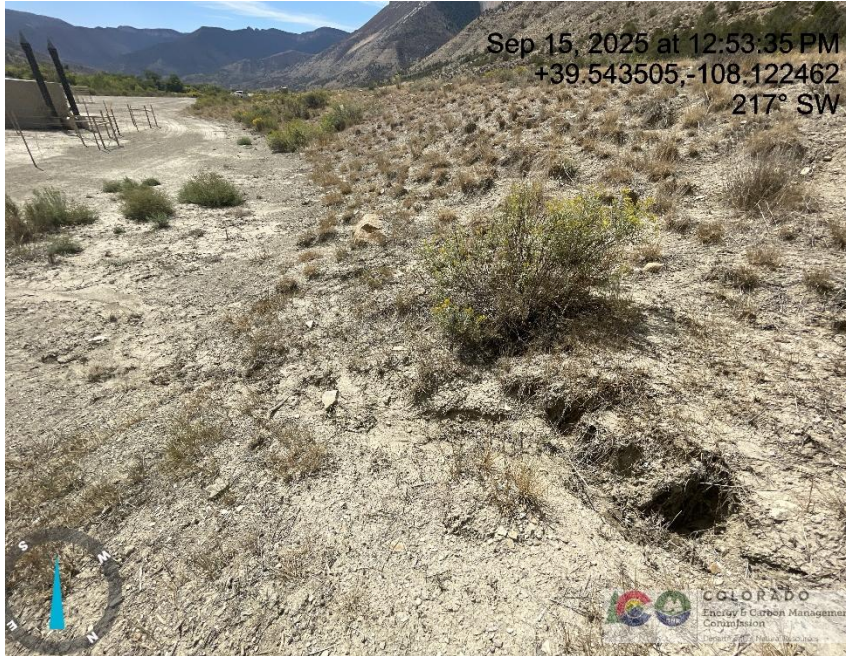
Photo # 8517 Erosion & transport of sediment onto location /insufficient BMP's
