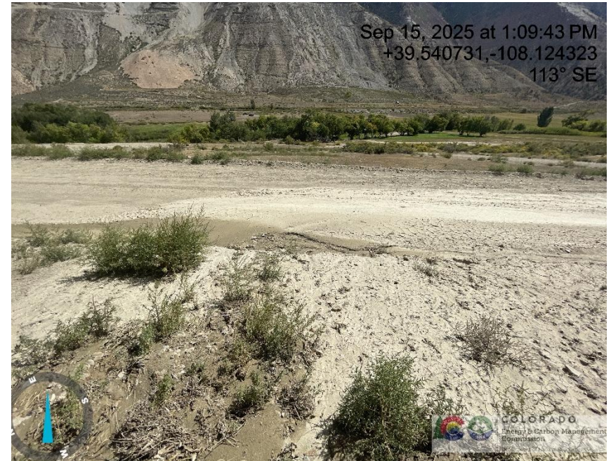
Photo # 8528 Erosion & transport of sediment onto lease road/insufficient BMP's (approximately 2/10th of a mile from entrance to location)
