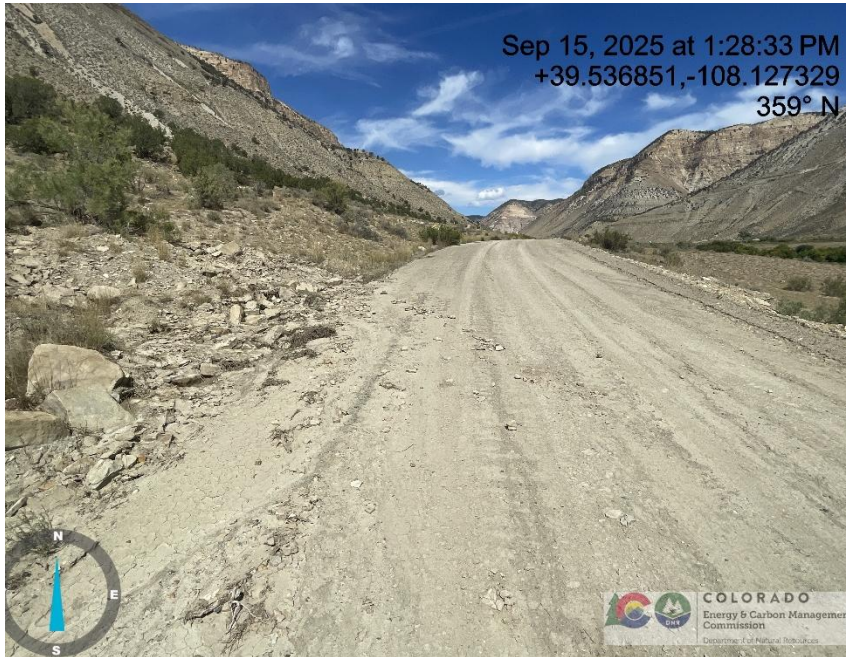
Photo # 8559 Erosion & transport of sediment onto lease road/insufficient BMP's (approximately 5/10th of a mile from entrance to location)
