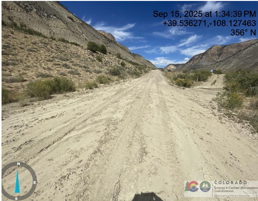
Photo # 8569 Erosion & transport of sediment onto lease road/insufficient BMP's (approximately 6/10th of a mile from entrance to location)
