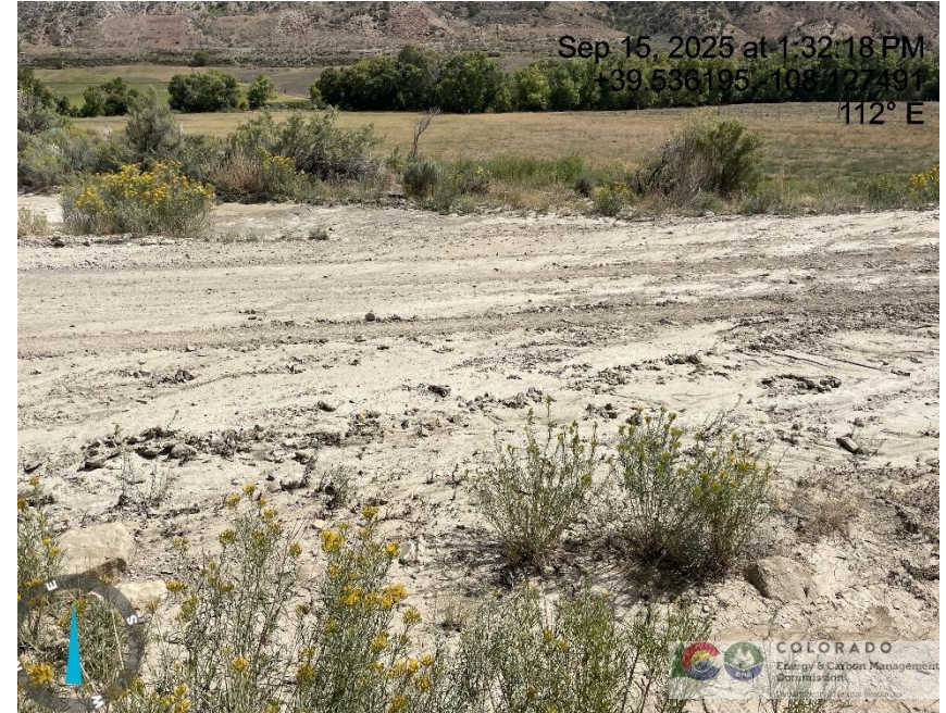
Photo # 8568 Erosion & transport of sediment onto lease road/insufficient BMP's (approximately 6/10th of a mile from entrance to location)
