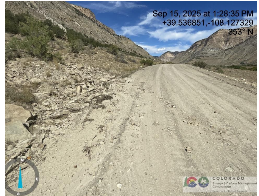
Photo # 8560 Erosion & transport of sediment onto lease road/insufficient BMP's (approximately 5/10th of a mile from entrance to location)
