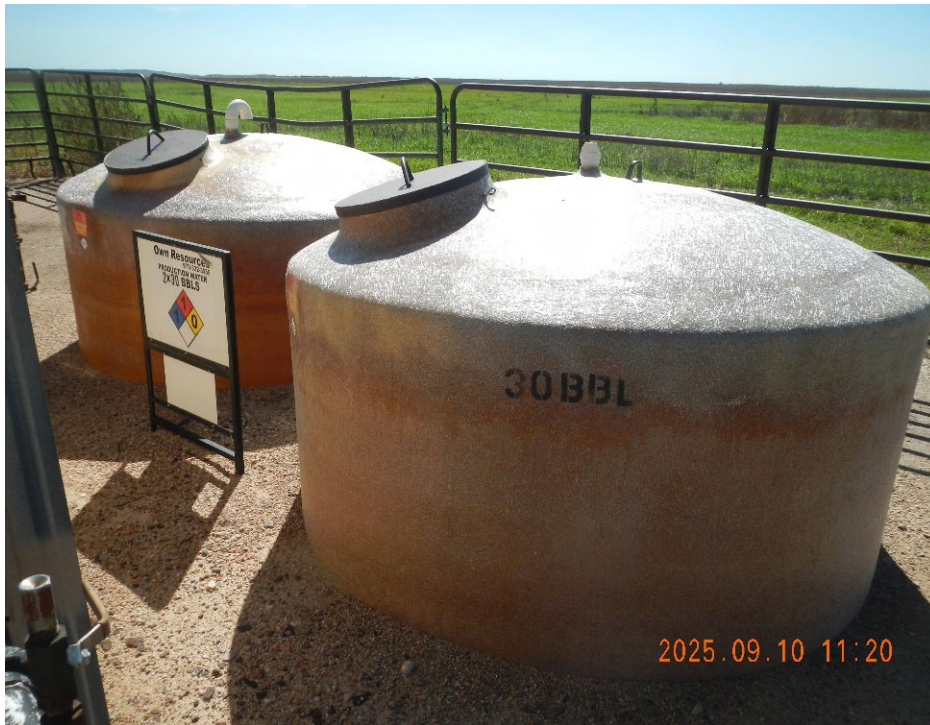
3. View of produced water tanks with sign.
