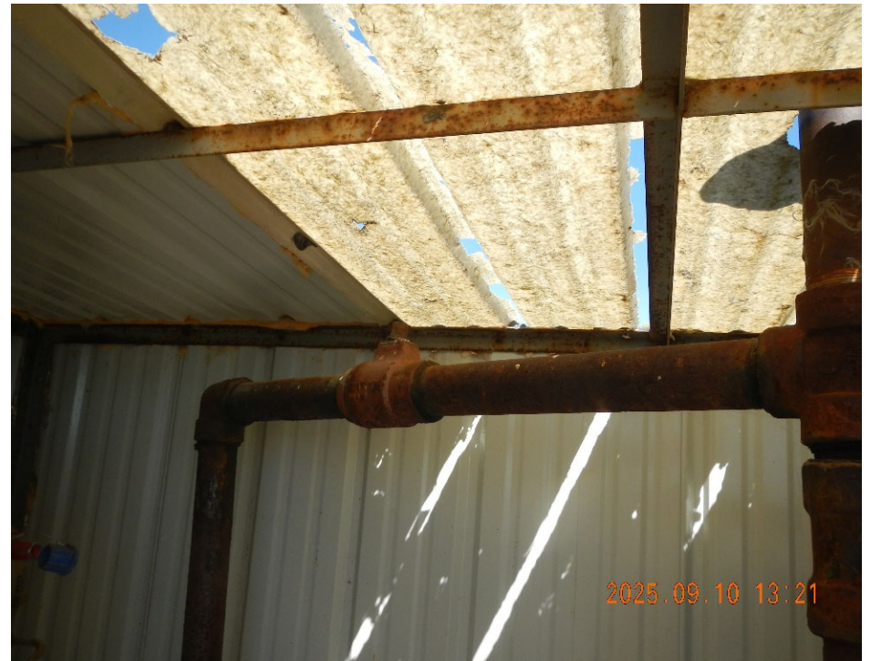
4. Meter shed roof damage.
