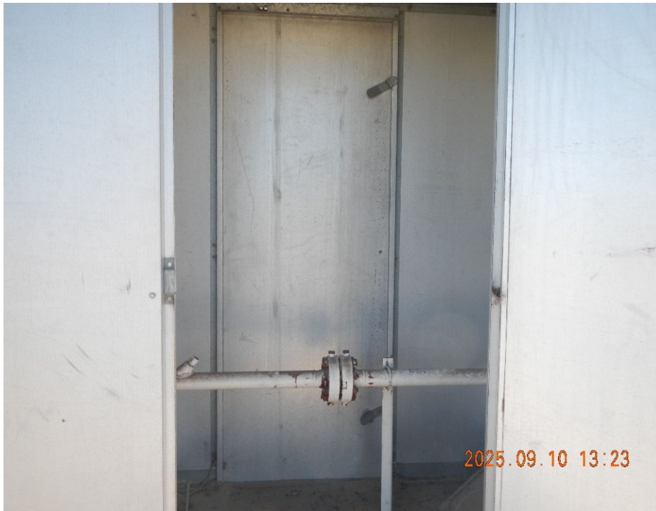
7. No gas meter on the inside of the abandoned flowline meter shed.
