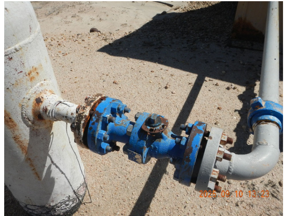
6. Closed valve on inlet.
