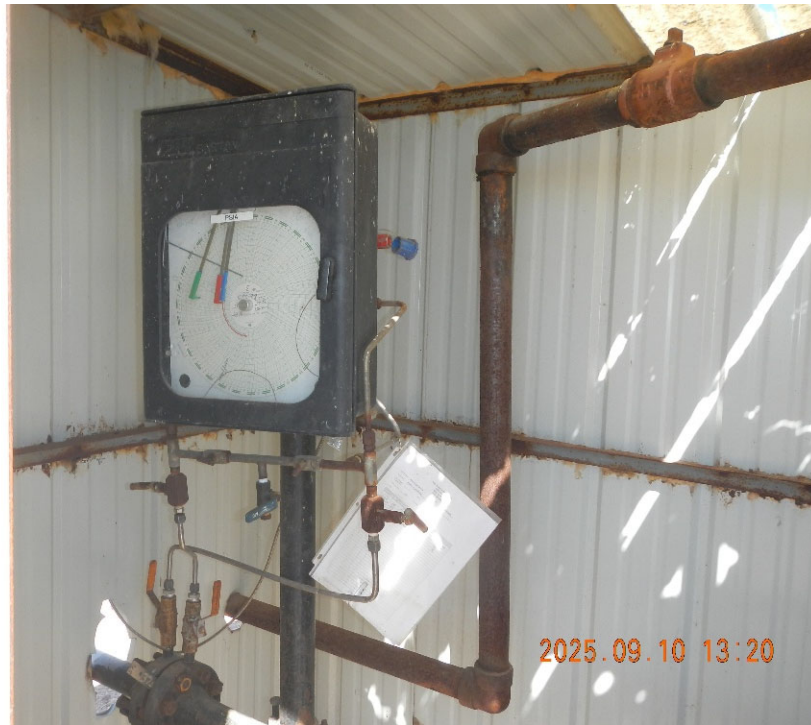
3. Gas Meter inside Meter Shed.
