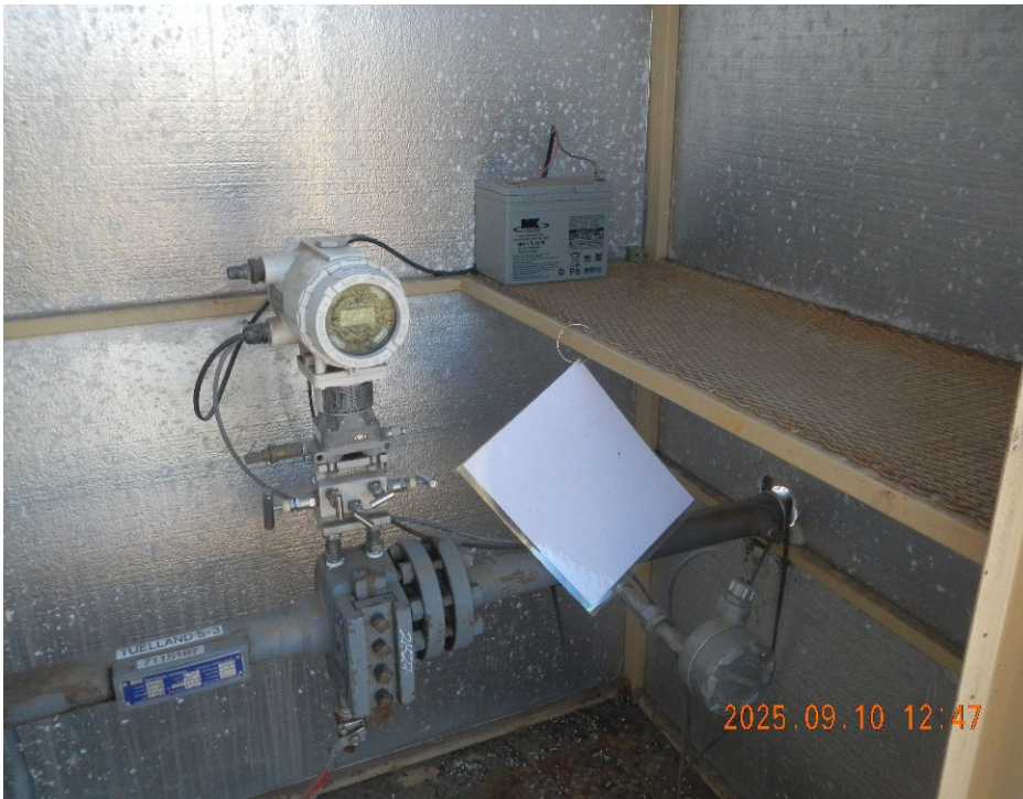
5. Gas meter inside meter shed.
