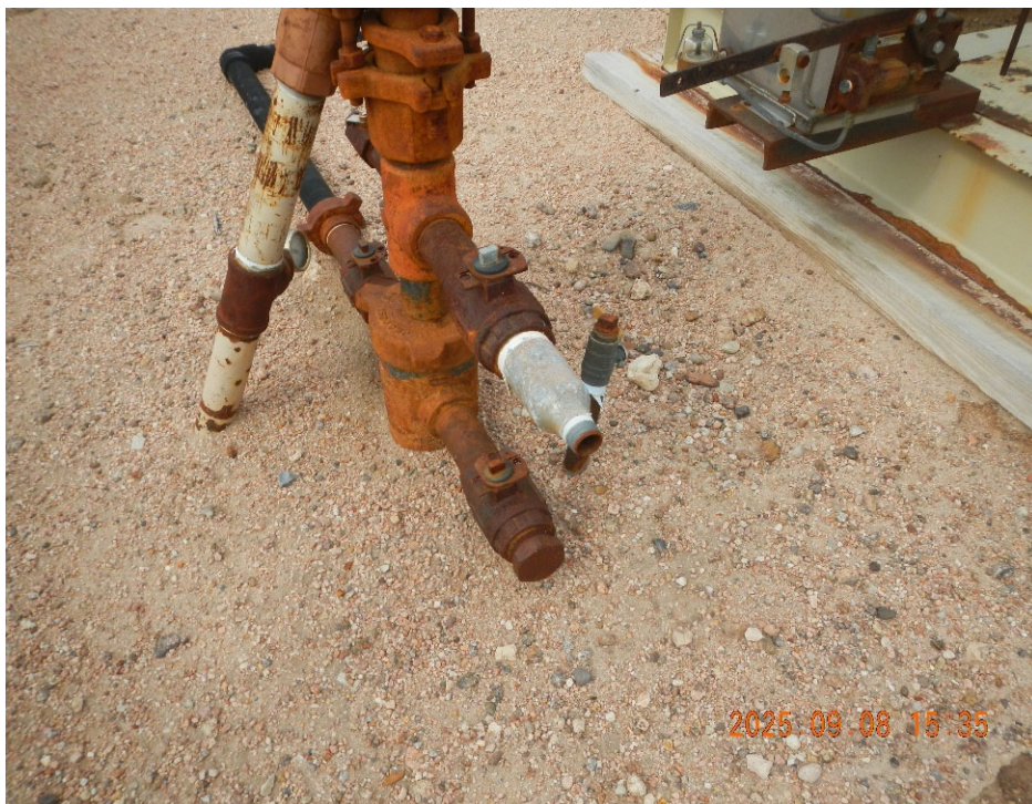
3. View of open ended line at wellhead.
