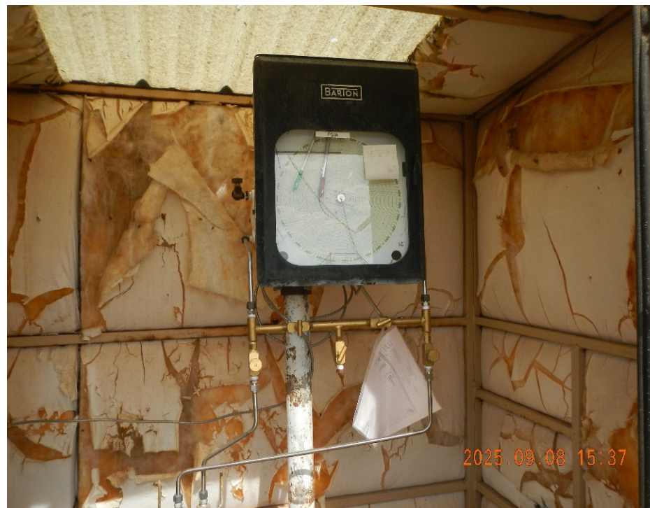
4. Gas Meter inside Meter Shed.
