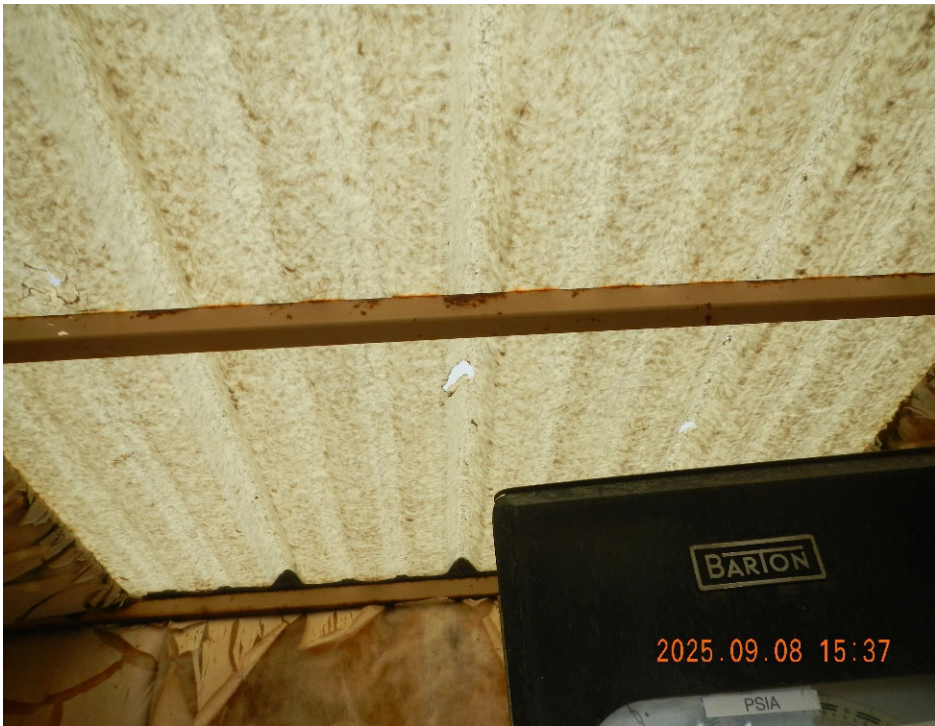
5. Meter Shed roof hail damage.
