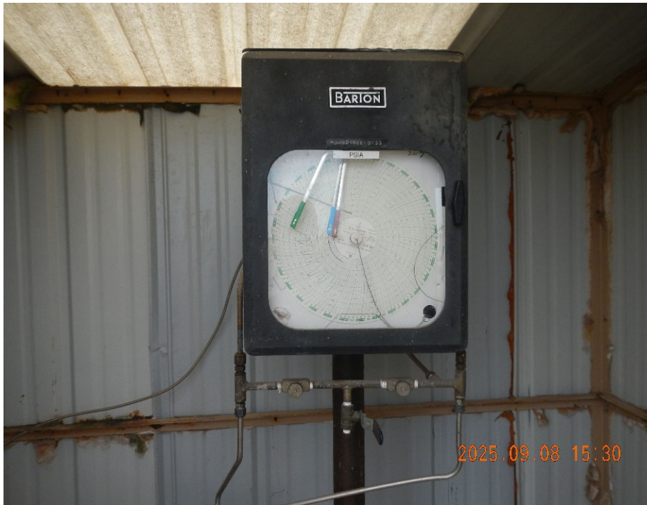
3. Gas Meter inside Meter Shed.
