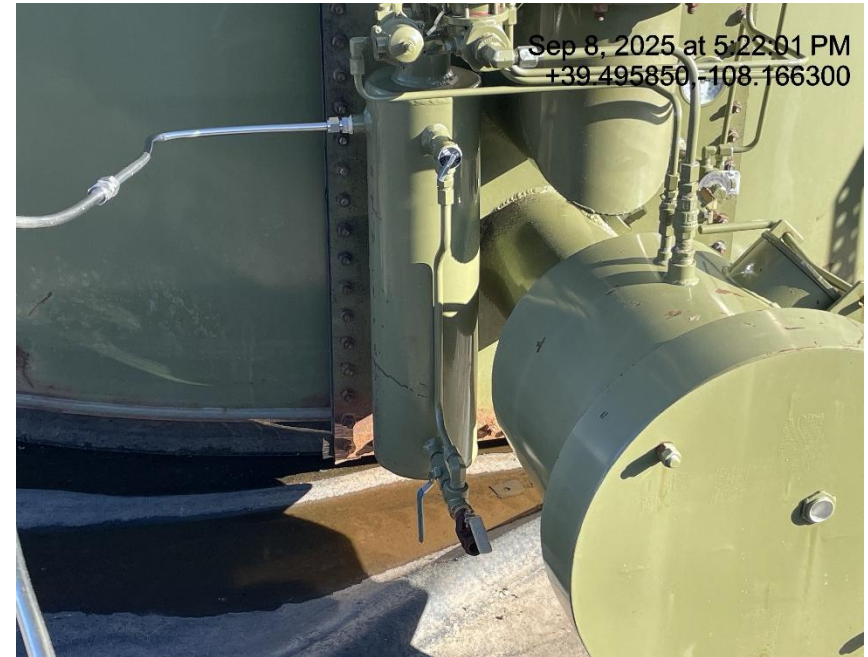
Photo # 7123 PRV vent line on tank burner does not comply with CECMC pressure safety device rules
