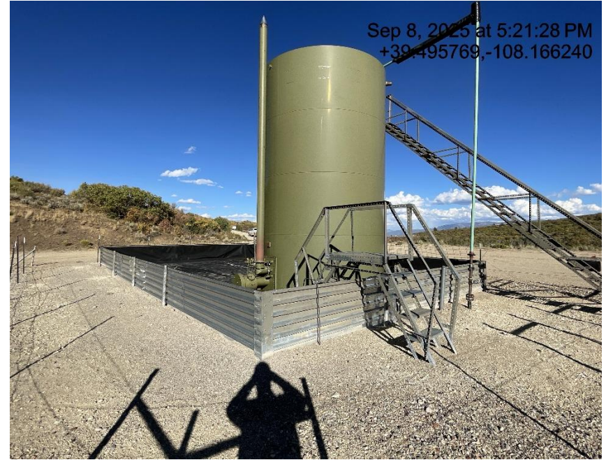
Photo # 7125 Tank battery lacks required signage
