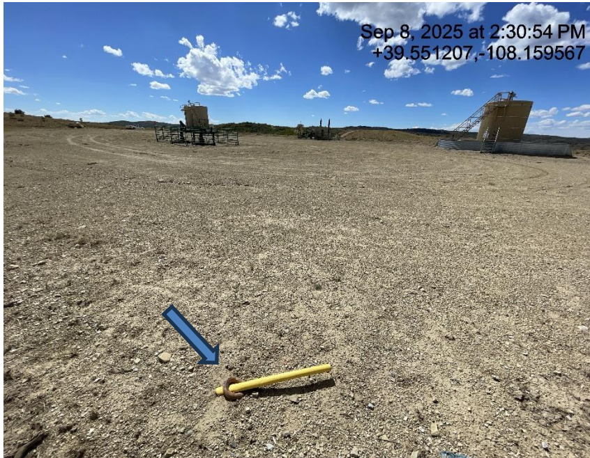
Photo # 6807 Improperly marked deadman
