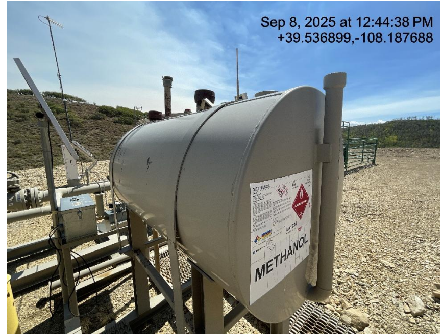
Photo # 6516 Chemical tank lacks required labeling
