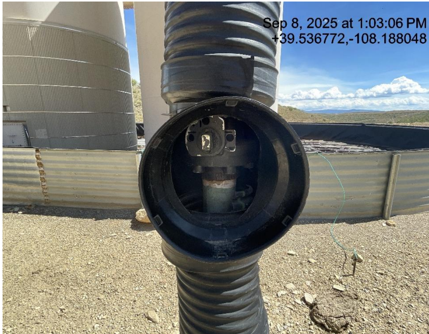
Photo # 6519 Flowline heating insulation open ended /wildlife hazard/available for entry by wildlife
