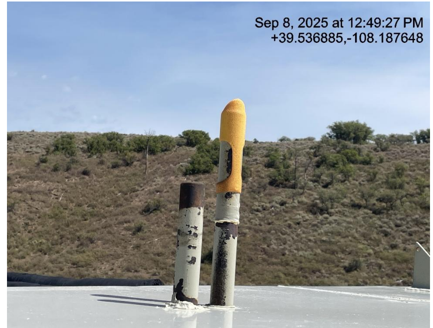
Photo # 6514 Rupture disc vent line does not comply with CECMC pressure safety device rules
