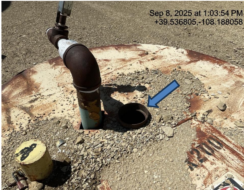
Photo # 6527 Opening on cellar cover/wildlife hazard /available for entry by wildlife
