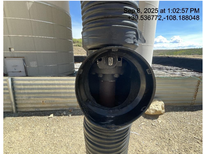
Photo # 6518 Flowline heating insulation open ended /wildlife hazard/available for entry by wildlife
