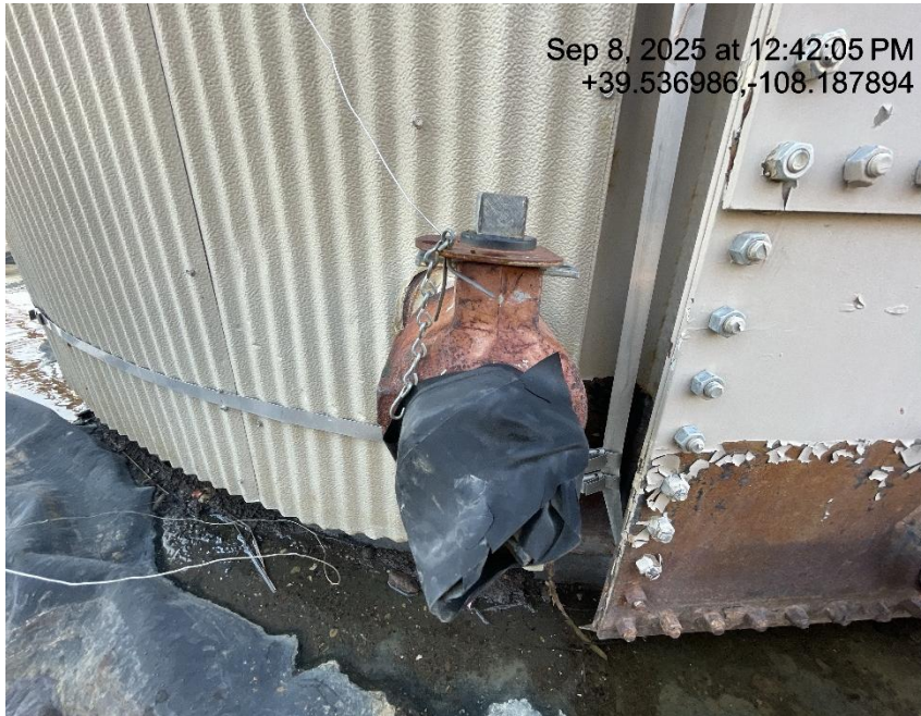
Photo # 6511 Open ended load line
