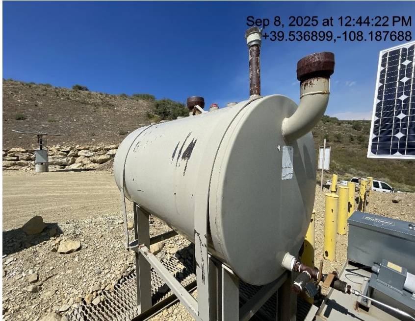
Photo # 6515 Chemical tank lacks required labeling
