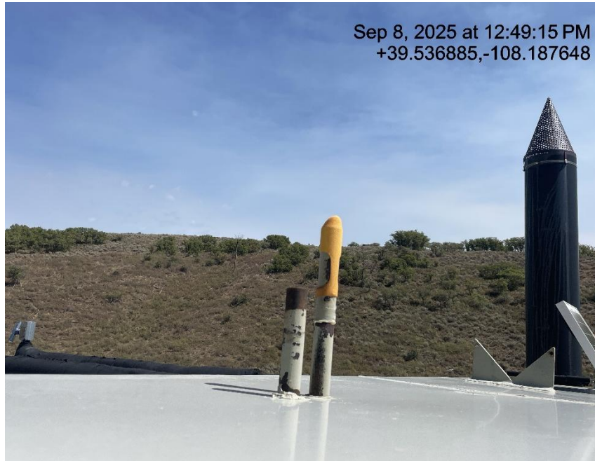
Photo # 6513 Rupture disc vent line does not comply with CECMC pressure safety device rules
