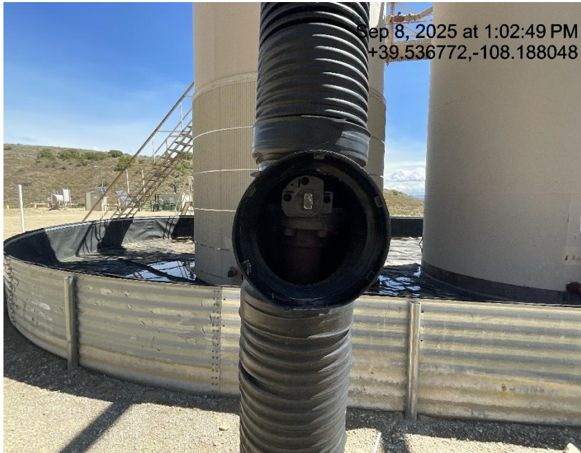
Photo # 6517 Flowline heating insulation open ended /wildlife hazard/available for entry by wildlife
