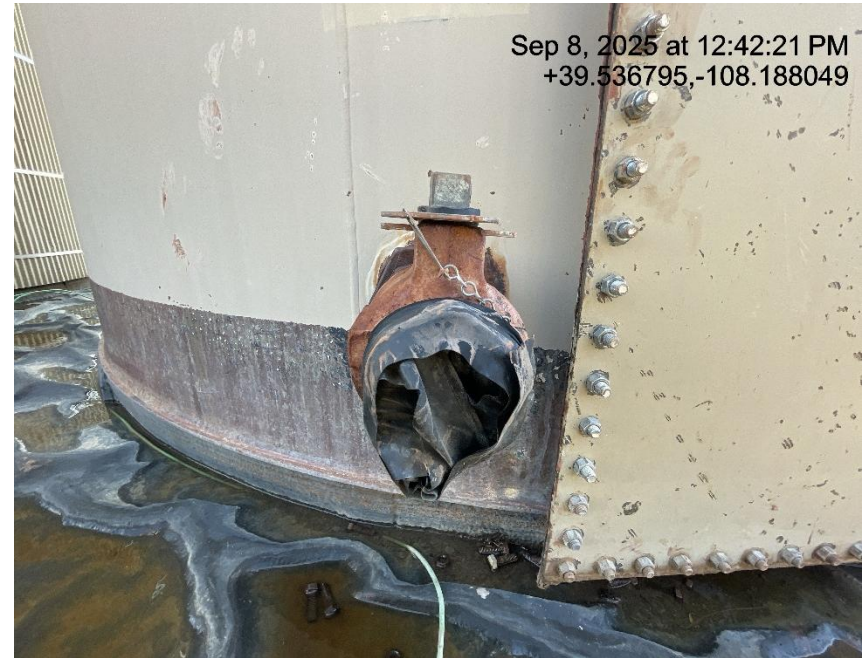
Photo # 6512 Open ended load line
