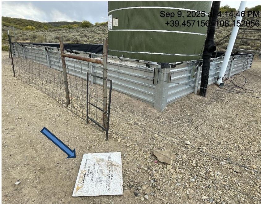
Photo # 7783 Battery sign laying on ground/not properly posted
