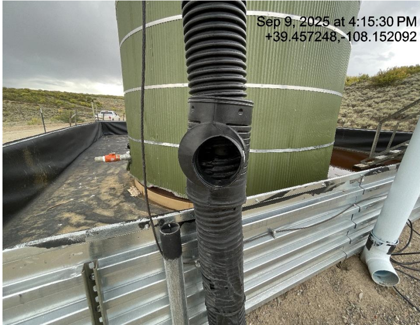
Photo # 7779 Flowline heating insulation open ended /wildlife hazard/available for entry by wildlife
