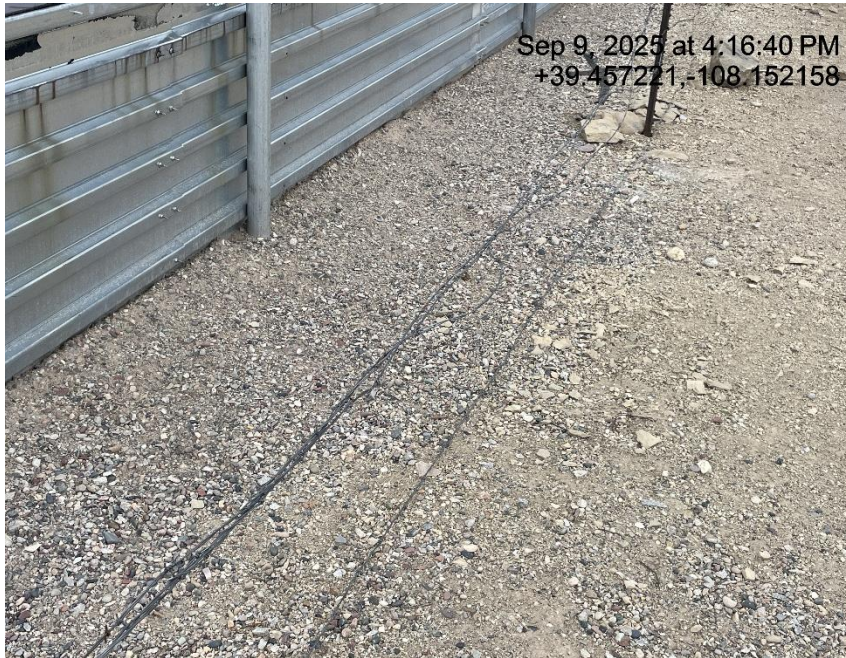
Photo # 7781 Barbed wire fence around tank battery needs maintenance/wildlife hazard
