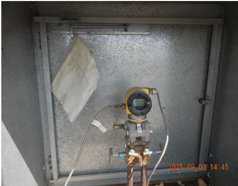
3. Gas Meter inside Meter Shed.
