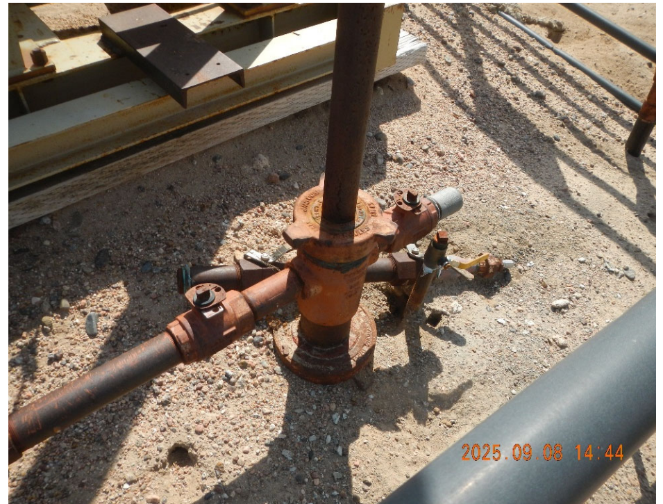
2. View of wellhead.
