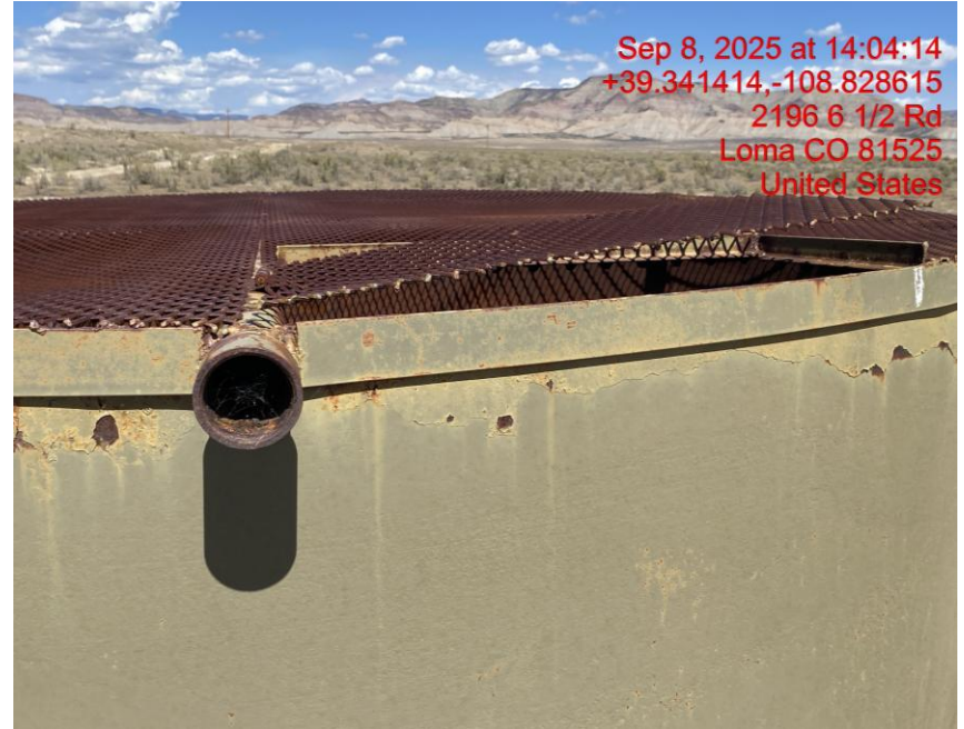
Wildlife Entry Hazard – Photo #00642
