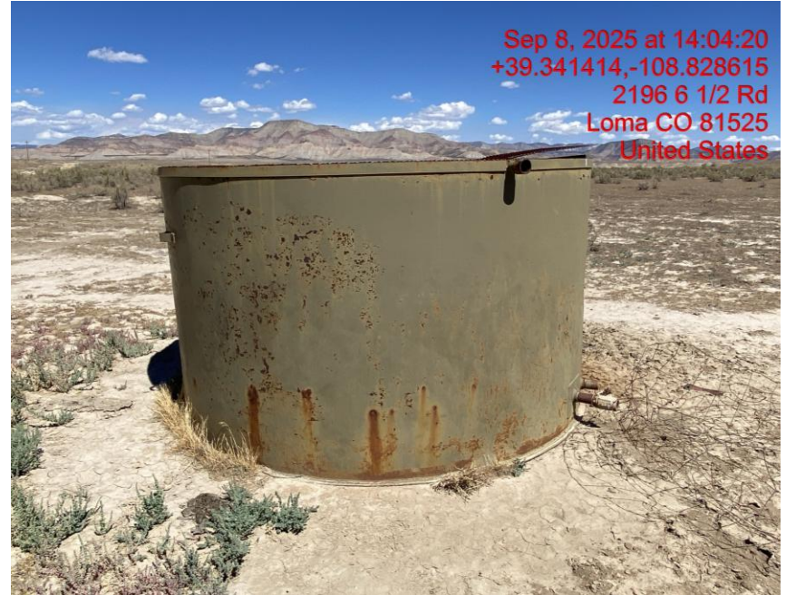
Location/Unused Equipment/No Tank Labels or Battery Sign Posted – Photo #00643
