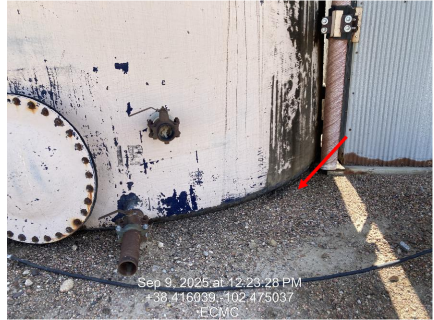
Photo 10 – Areas of impacted soils
