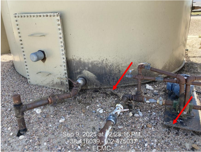
Photo 9 – Areas of impacted soils
