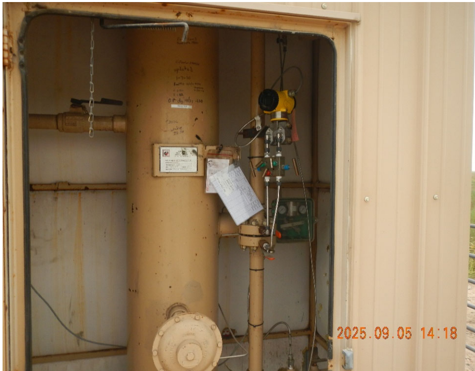
3. Vertical Separator and Gas Meter inside Meter Shed.
