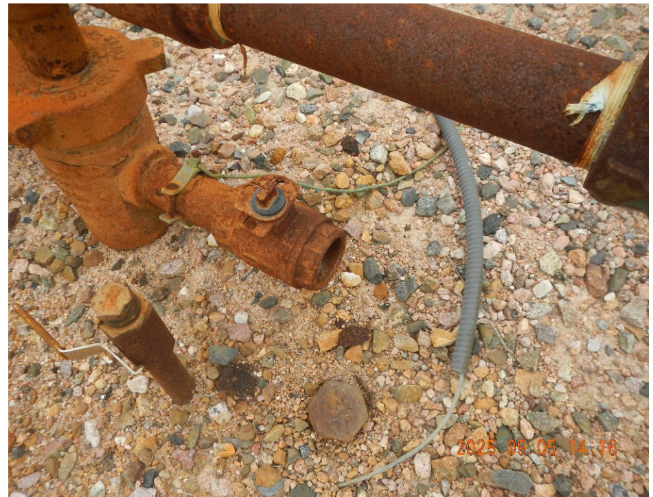
2. View of open-ended line at wellhead.
