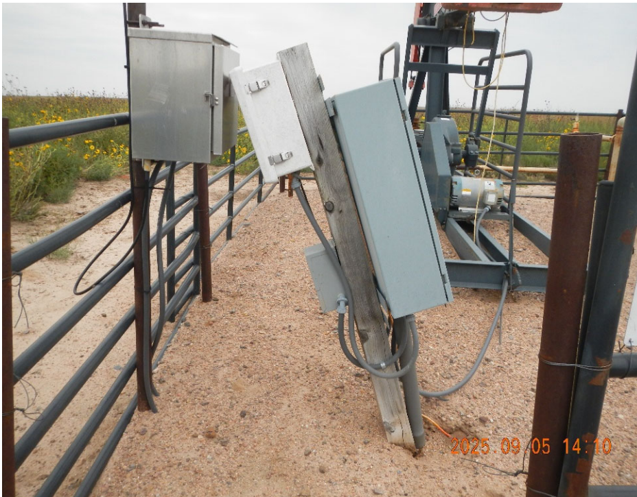
3. View of pump control panels leaning on radio battery box.
