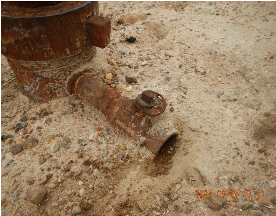
3. View of surface casing open to atmosphere on wellhead.
