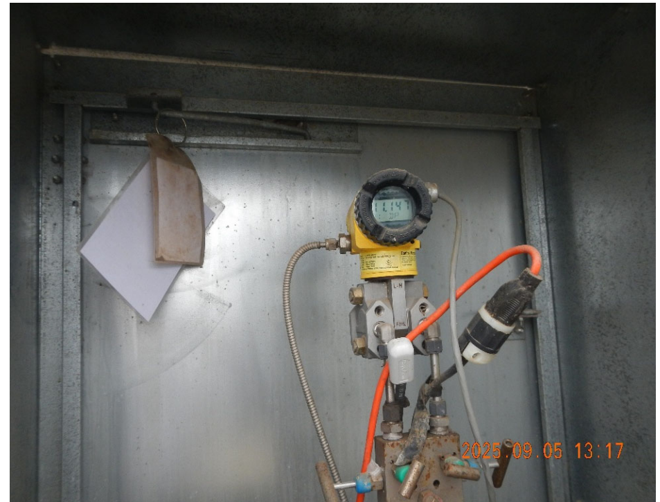
4. Gas meter inside meter shed.
