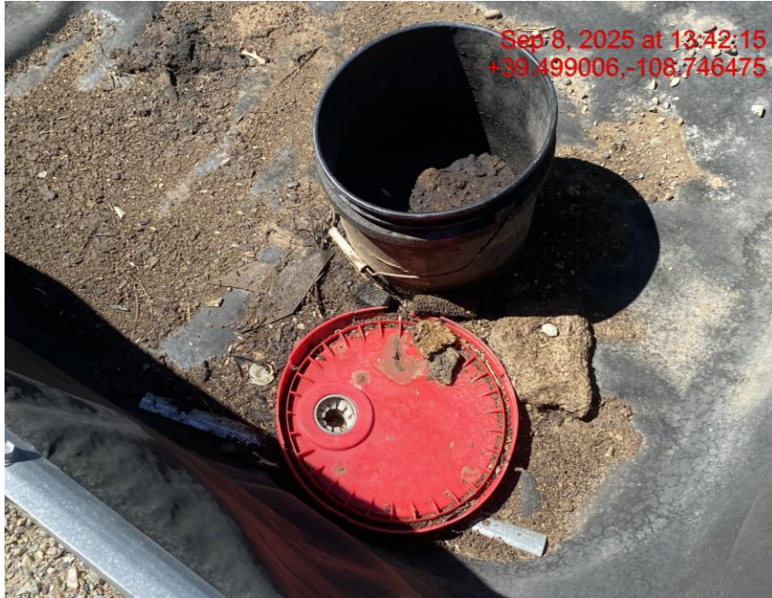
Trash/Debris In Secondary Containment – Photo #00627
