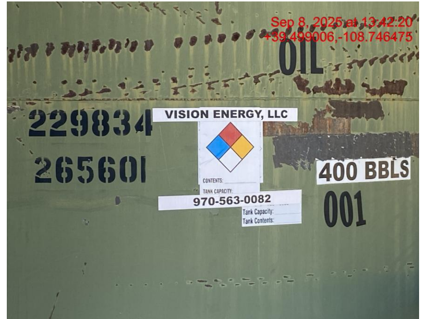
Labels Missing Required Information – Photo #00628
