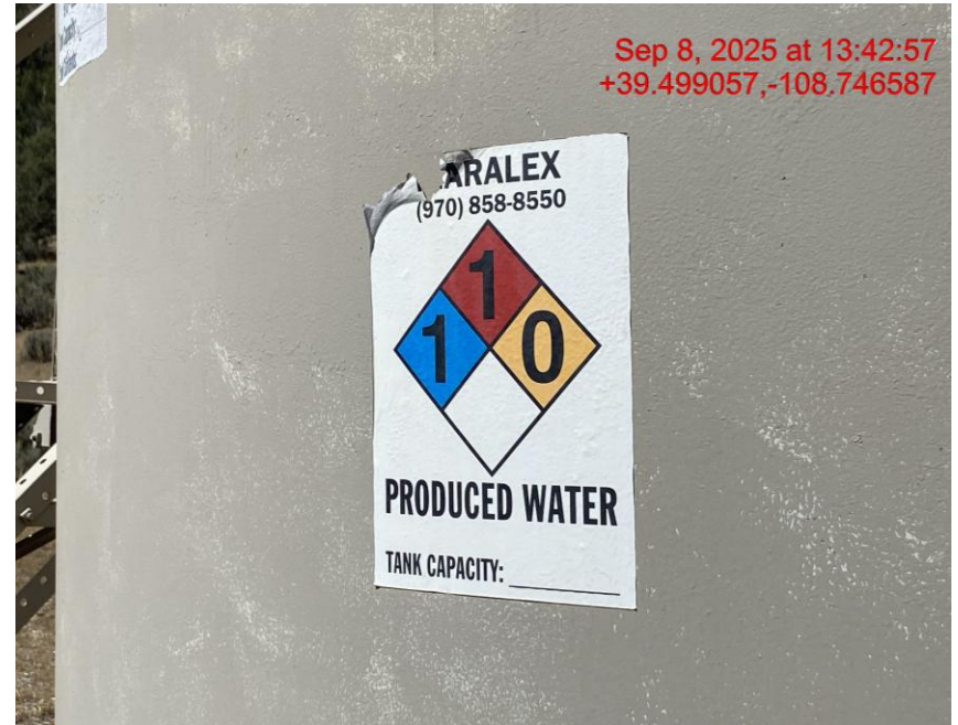
Labels Missing Required Information – Photo #00630
