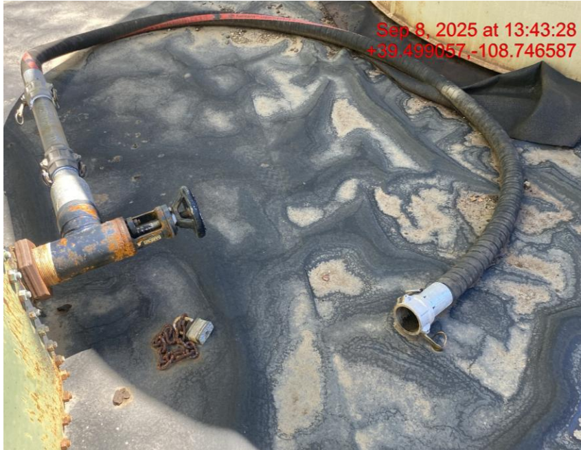
Wildlife Entry Hazard – Photo #00632
