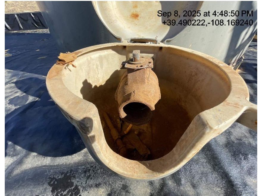
Photo # 6974 Open ended load line
