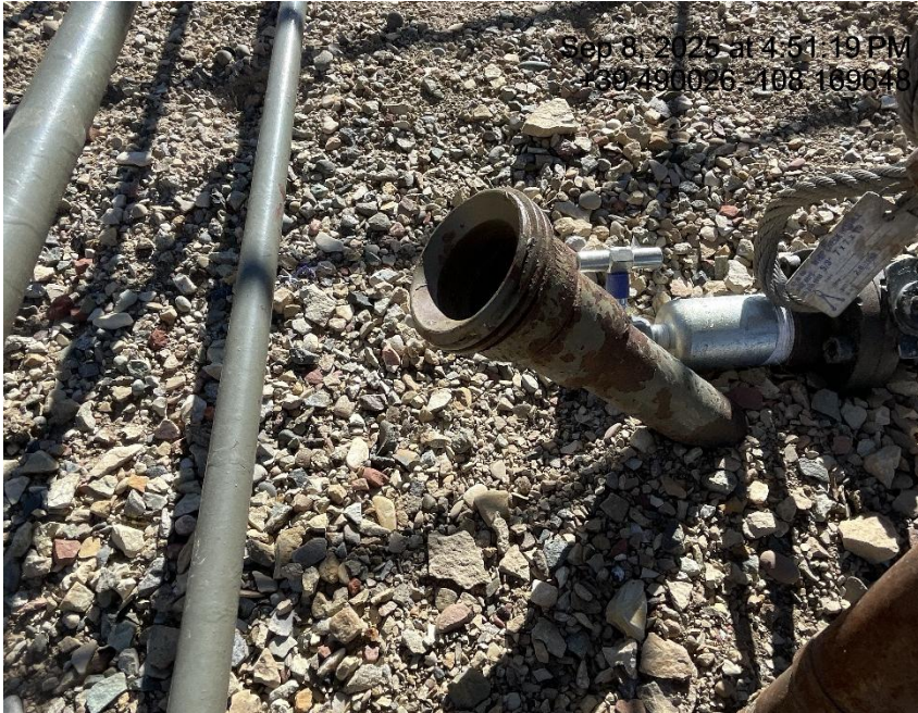
Photo # 6975 Open ended piping near wellhead/wildlife hazard
