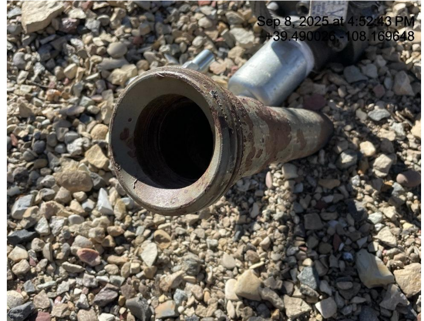
Photo # 6976 Open ended piping near wellhead/wildlife hazard
