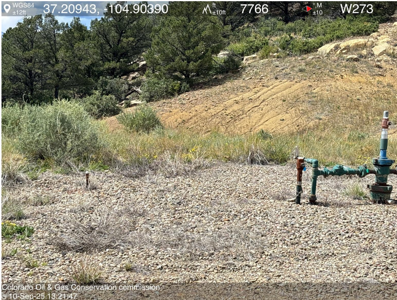
PHOTO 3: UNUSED EQUIPMENT (1" RISER NEAR WELLHEAD). WELL HAS BEEN IN TA STATUS FOR OVER 10 YEARS, RISER NEEDS TO BE REMOVED PER RULE 606. CA DATE 10/10/2025.
