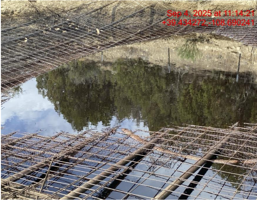
Insufficient Netting Over Pit – Photo #00575
