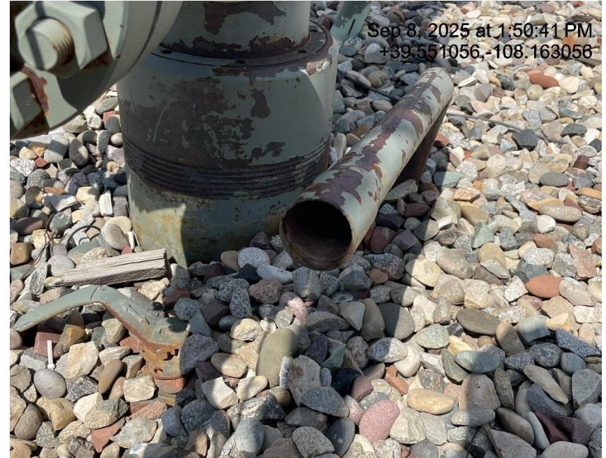
Photo # 6653 Open ended piping near wellhead/wildlife hazard
