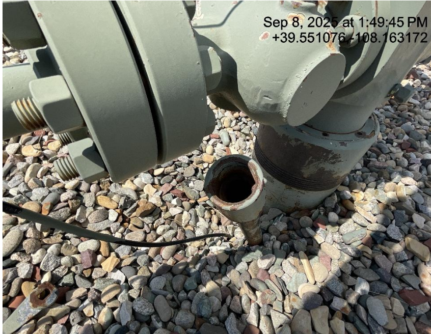
Photo # 6652 Open ended piping near wellhead/wildlife hazard
