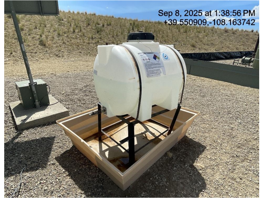
Photo # 6645 Unused equipment
