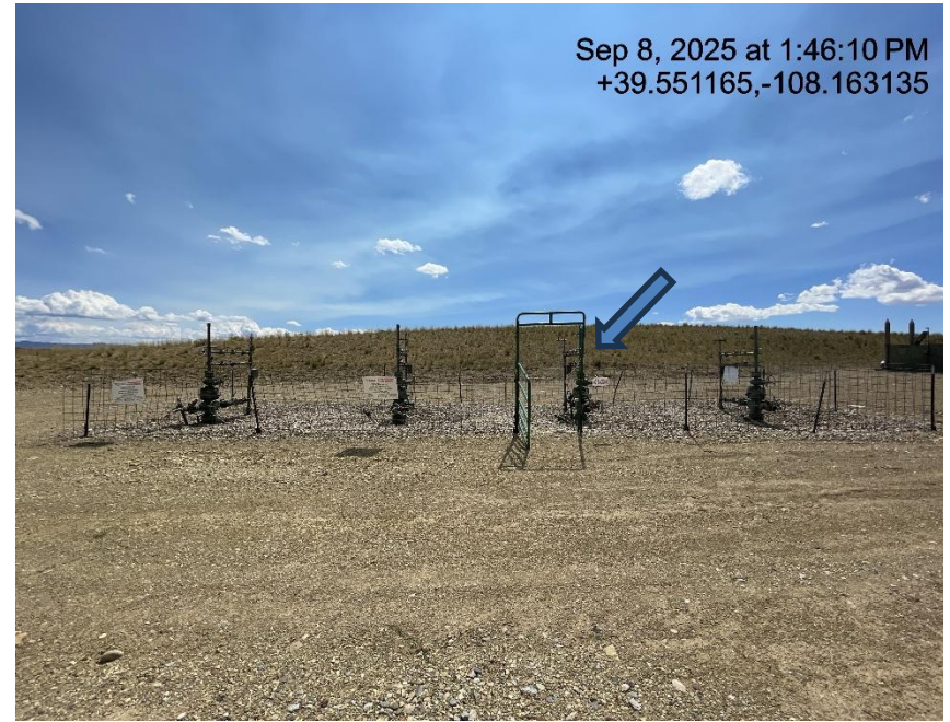
Photo # 6649 CHEVRON 275-1 well lacks required signage
