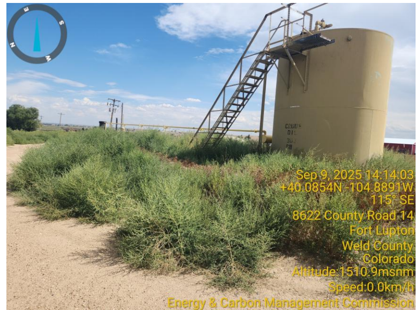
Photo 6 Tank Battery is overrun with vegetation ..
