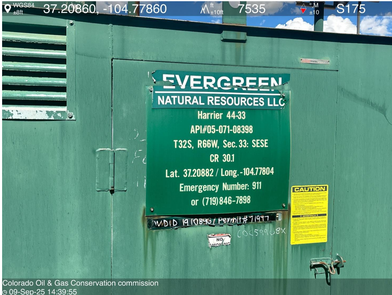
PHOTO 1: WELL SIGN IS ON THE SOUTHSIDE OF THE METER HOUSE WHICH IS VERY CLOSE TO THE SOUTH HIGH BANK OF THE CUT. PER RULE 605 THIS SIGN SHOULD BE PLACED IN AN EASY TO READ FROM A DISTANCE (SHOULD BE ON THE ENTRANCE OF LOCATION SIDE OF METER HOUSE OR AT LEAST THE LOCATION SIDE OF THE METER HOUSE).
