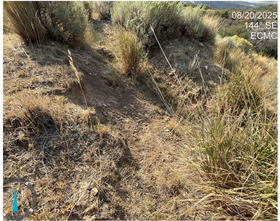
Photo 14. Photos 12-14 taken on the Fill slope on the western portion of the Location, illustrating rill and gully erosion, undercutting vegetation.
