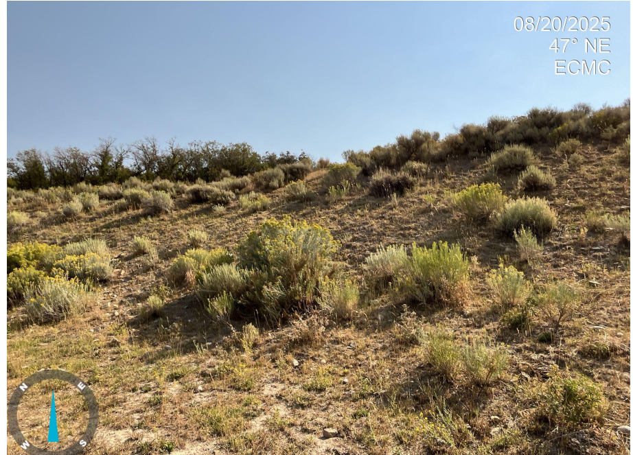
Photo 6. Photos 6-9 taken of the cut slope on the eastern portion of the Location. Photos illustrate that some areas remain bare with vegetation, which has led to destabilization and erosion on the cut slope.
