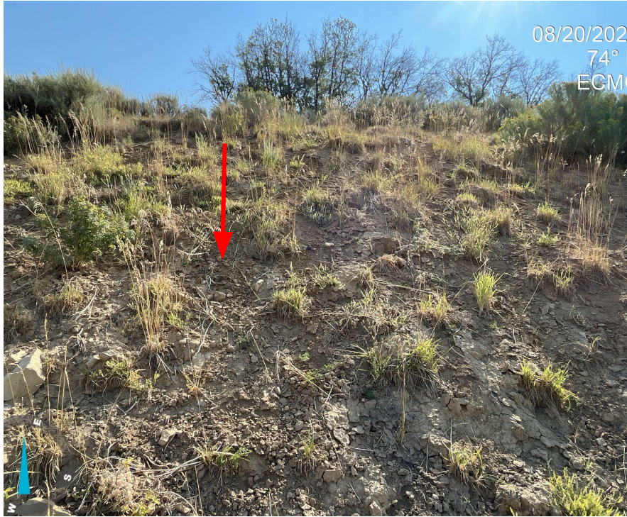
Photo 7. See comments under Photo 6. Red arrow indicates where rill erosion has started to occur.
