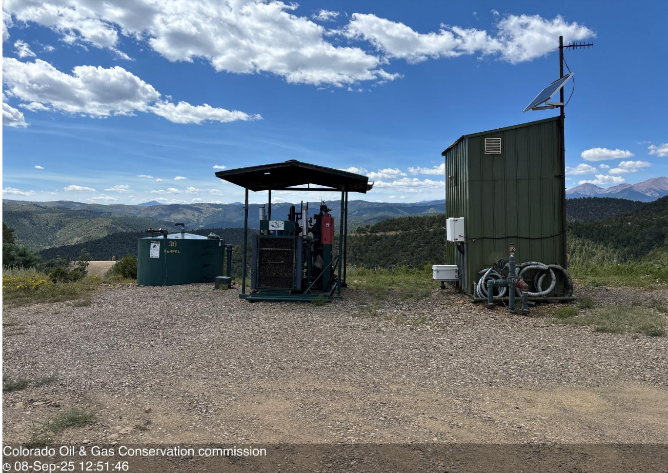
PHOTO 3: WELLHEAD AND EQUIPMENT.
