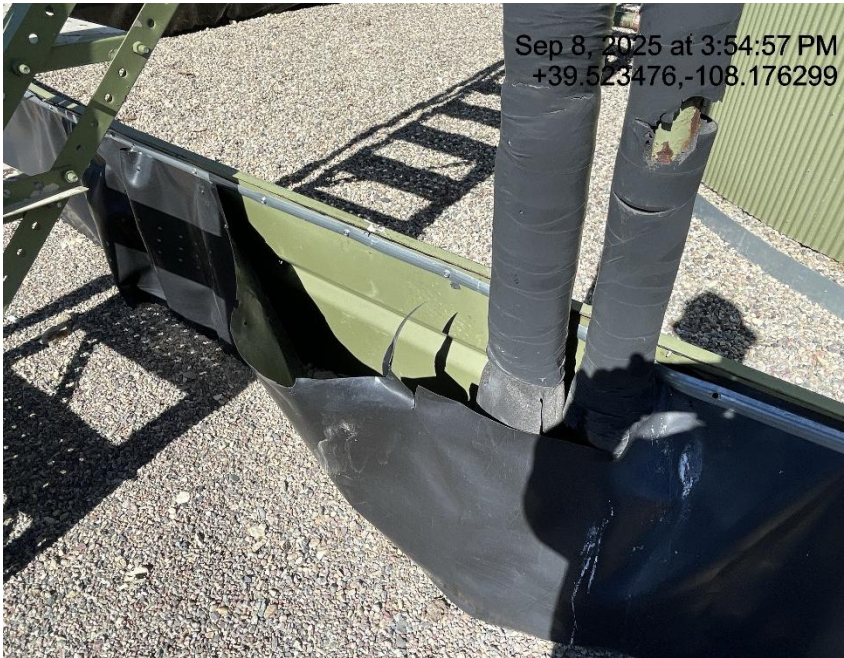
Photo # 6901 Secondary containment liner damaged/needs maintenance
