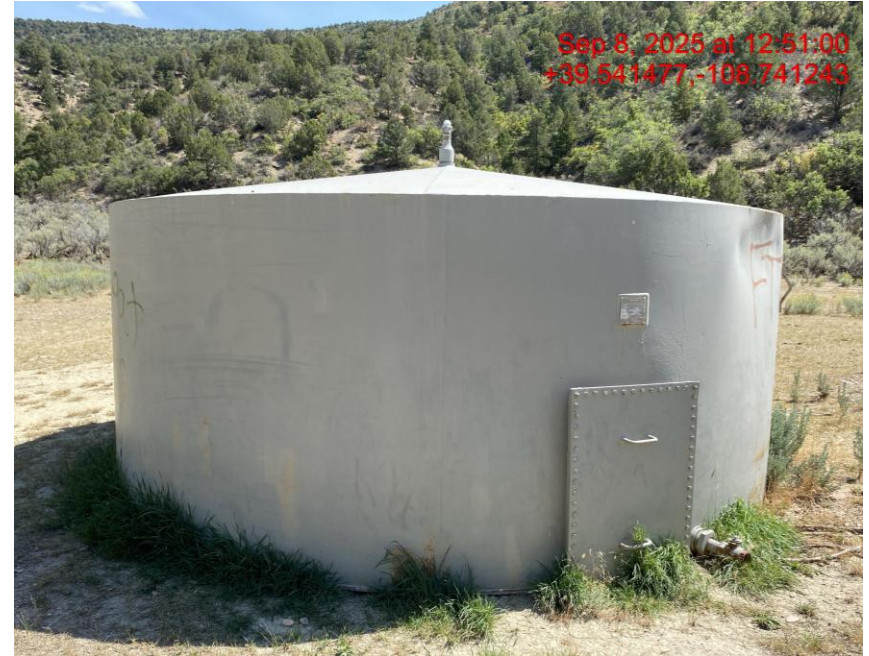
Unused Equipment/Weeds – Photo #00599
