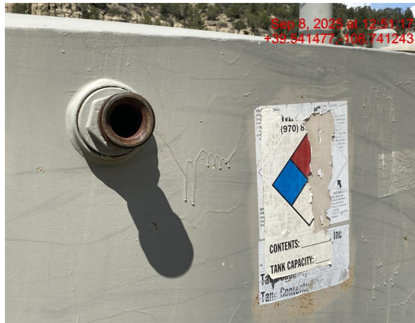
Wildlife Entry Hazard – Photo #00600
