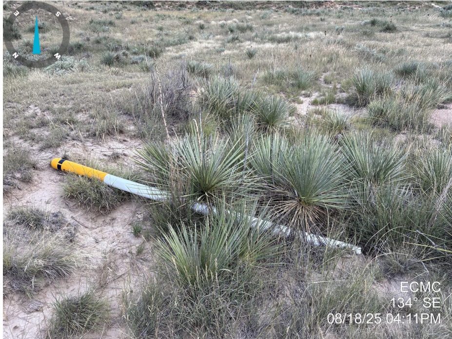
Photo 7. Photo taken from the access road, facing southeast. Photo illustrates midstream equipment that has fallen over.
