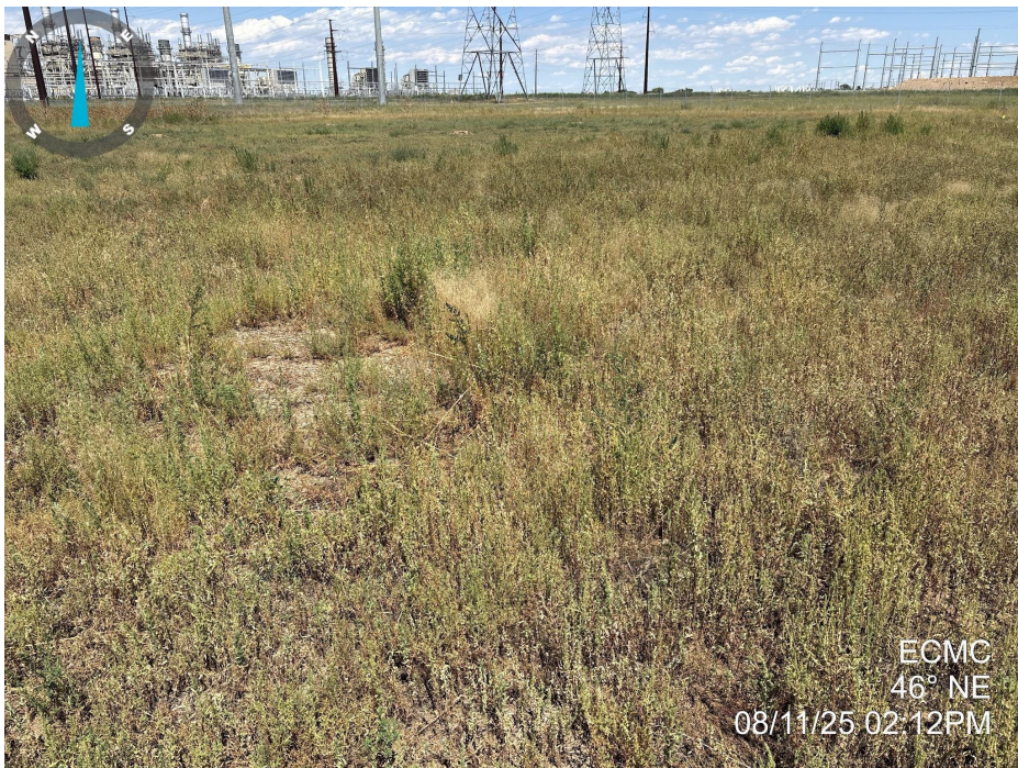
Photo 5. Photo taken of the tank battery location, facing northeast. Photo illustrates that final reclamation activities have taken place, but vegetation has not established to Rule 1004 standards. Weedy annual vegetation including kochia ( Bassia scoparia ) and cheatgrass ( Bromus tectorum ) dominates the location.
