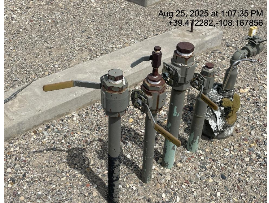
Photo # 3853 Unused flowlines lack lockout tagout (OOSLAT)
