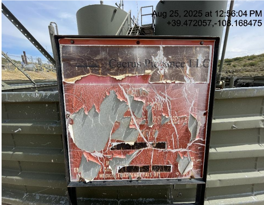
Photo # 3846 Battery sign damaged & illegible
