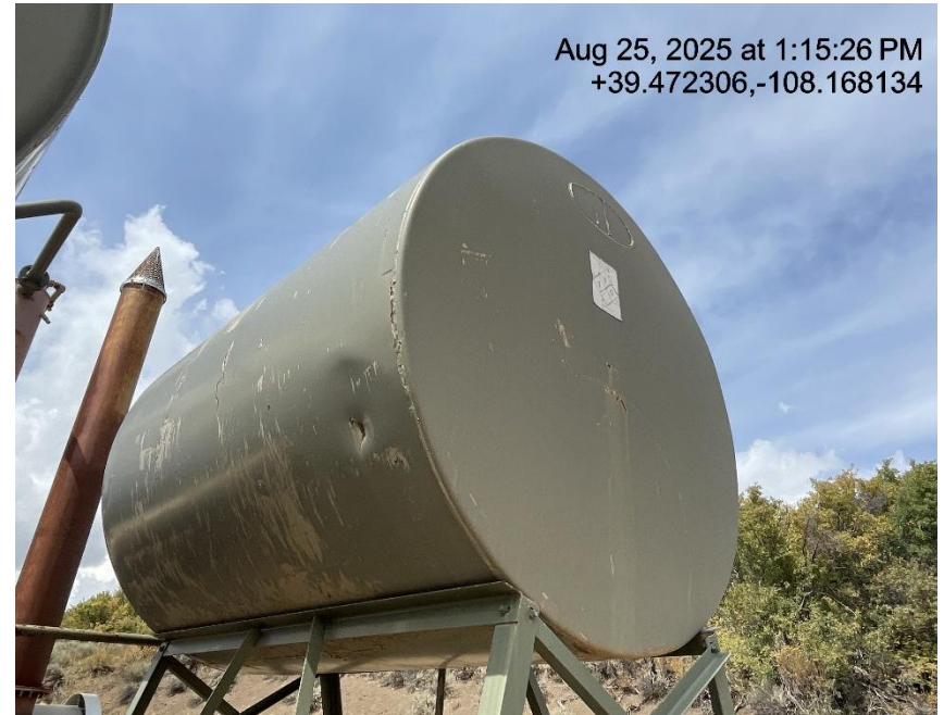
Photo # 3857 Chemical tank lacks required labeling
