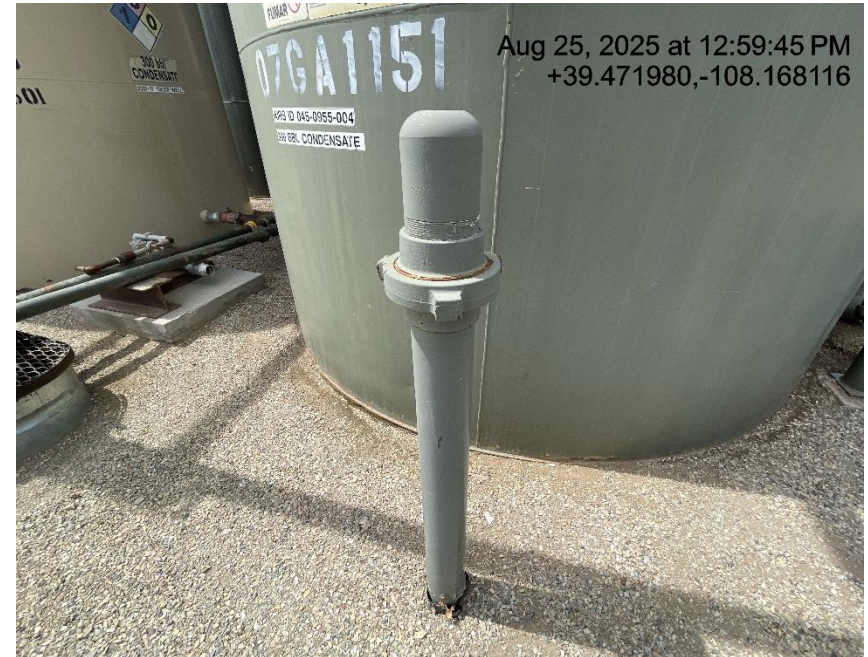
Photo # 3849 Unused flowline lacks lockout tagout (OOSLAT)
