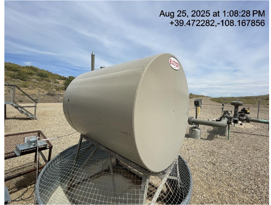
Photo # 3855 Chemical tank lacks required labeling
