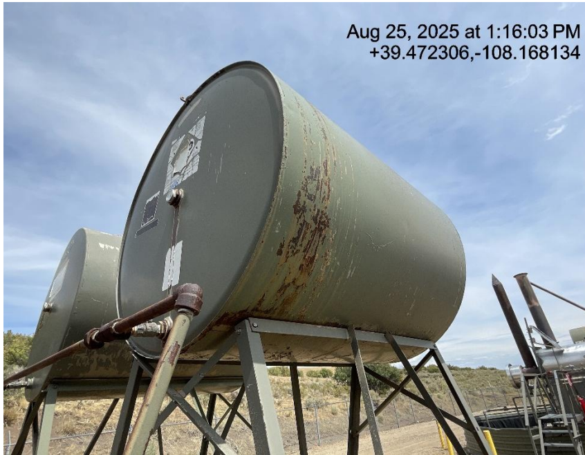
Photo # 3858 Chemical tank lacks required labeling
