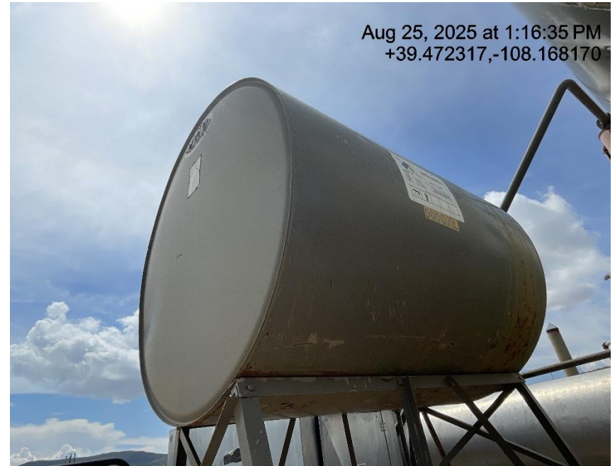
Photo # 3859 Chemical tank lacks required labeling
