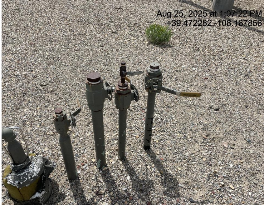
Photo # 3852 Unused flowlines lack lockout tagout (OOSLAT)
