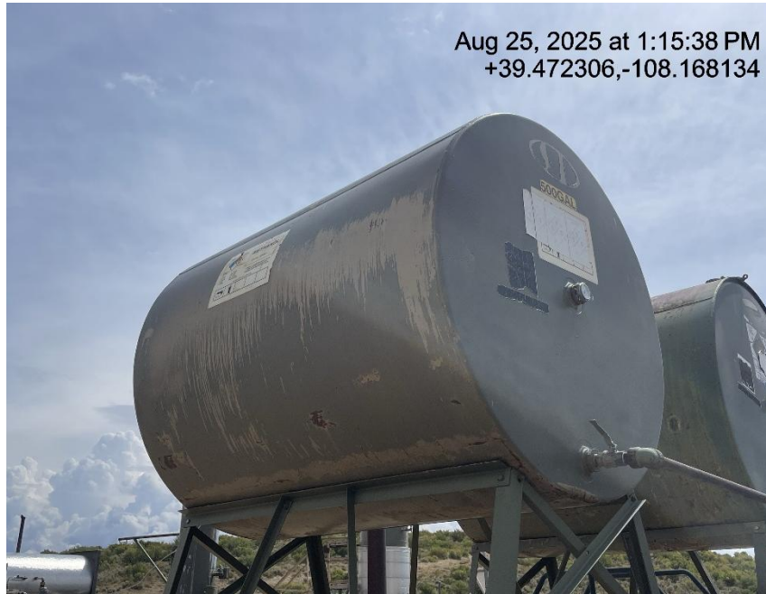
Photo # 3856 Chemical tank lacks required labeling
