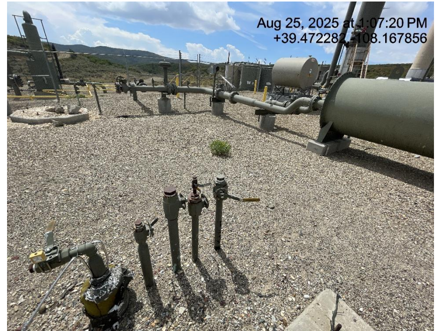
Photo # 3851 Unused flowlines lack lockout tagout (OOSLAT)
