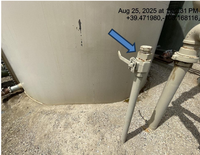
Photo # 3850 Unused flowline lacks lockout tagout (OOSLAT)
