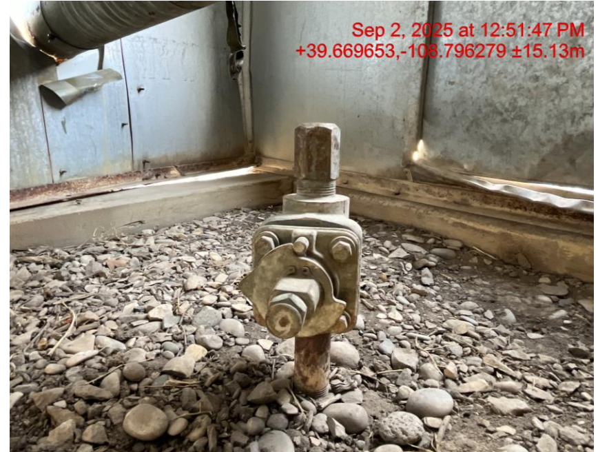
Photo # 2837 Unused flowline in meter house lacks lockout tagout (OOSLAT) Same flowline from other side
