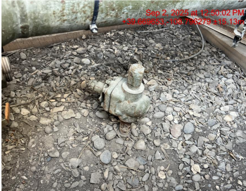
Photo # 2834 Unused flowline in meter house lacks lockout tagout (OOSLAT)
