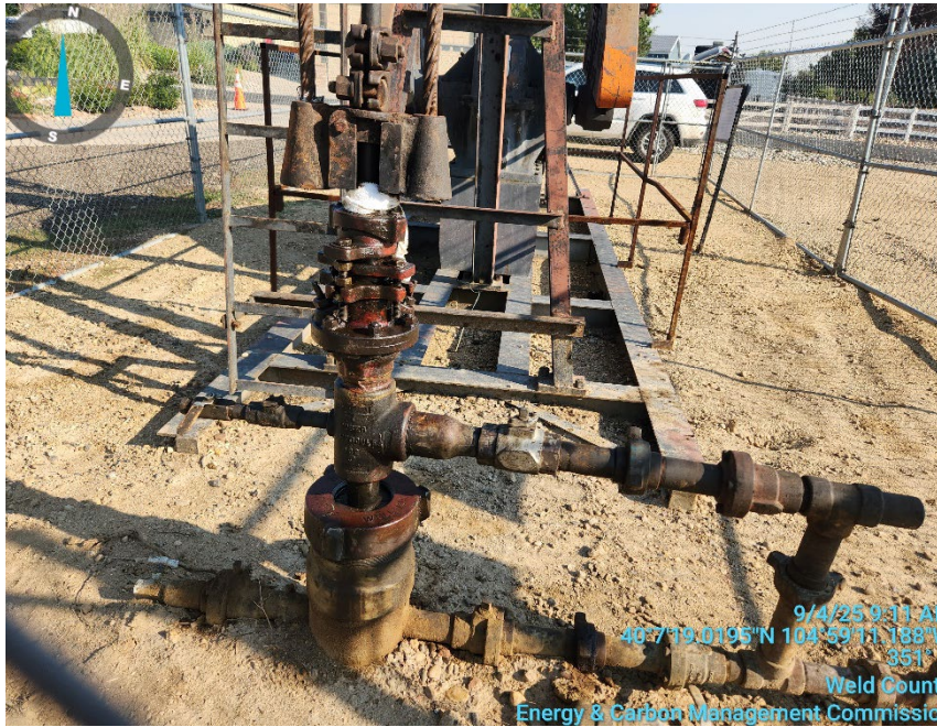
Photo 3: Location of leak
