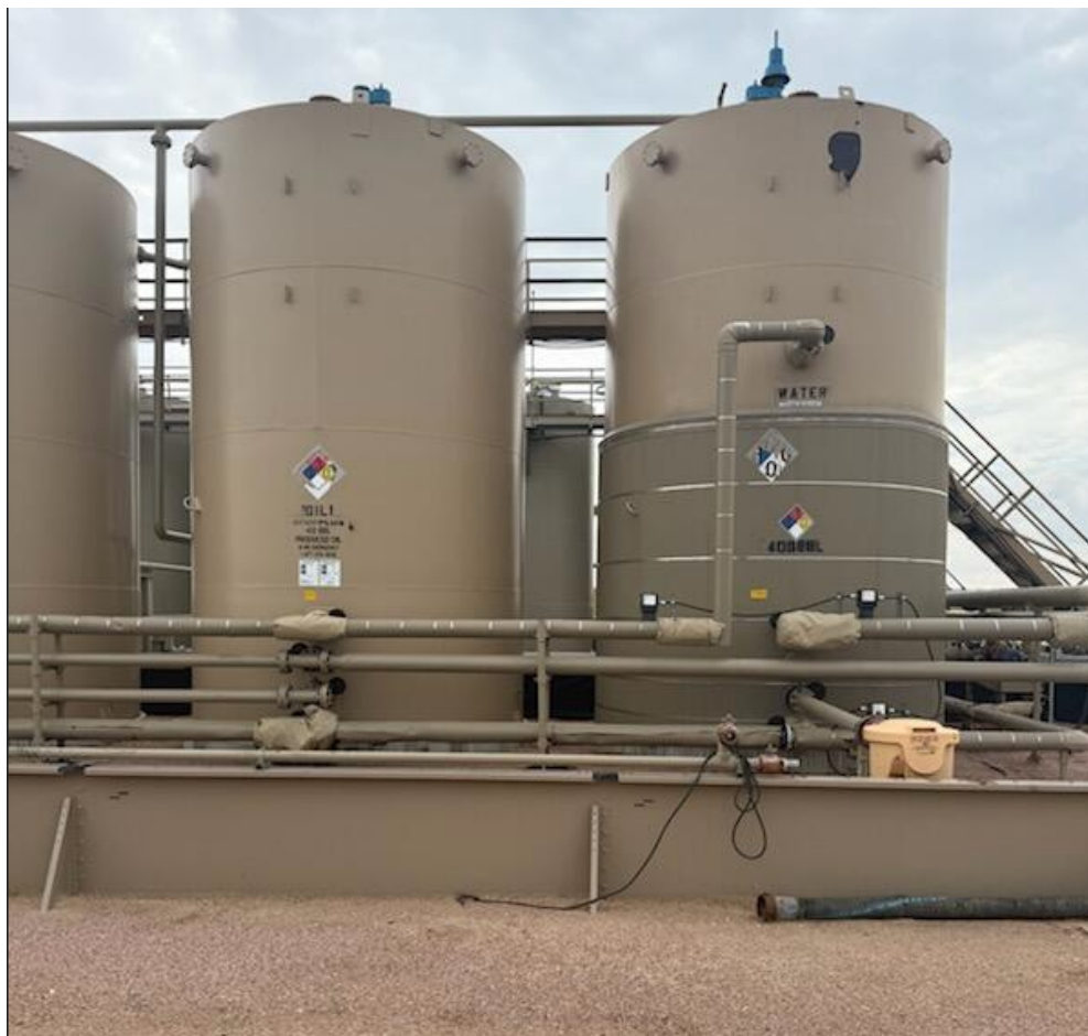
NFPA placards on all crude and produced water tanks replaced.
