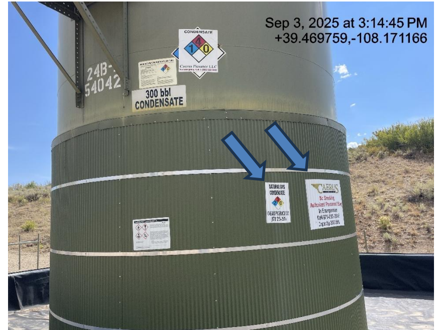
Photo # 6015 Tank labels have previous operators name/not in compliance with CECMC Rule 605
