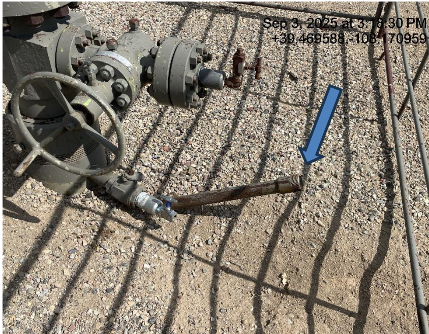
Photo # 6012 Open ended pipe at wellhead/wildlife hazard
