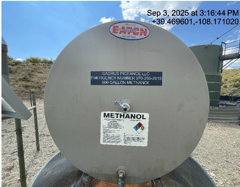
Photo # 6014 Tank label has previous operators name/not in compliance with CECMC Rule 605
