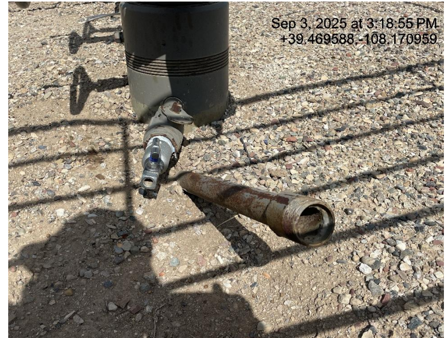
Photo # 6013 Open ended pipe at wellhead/wildlife hazard
